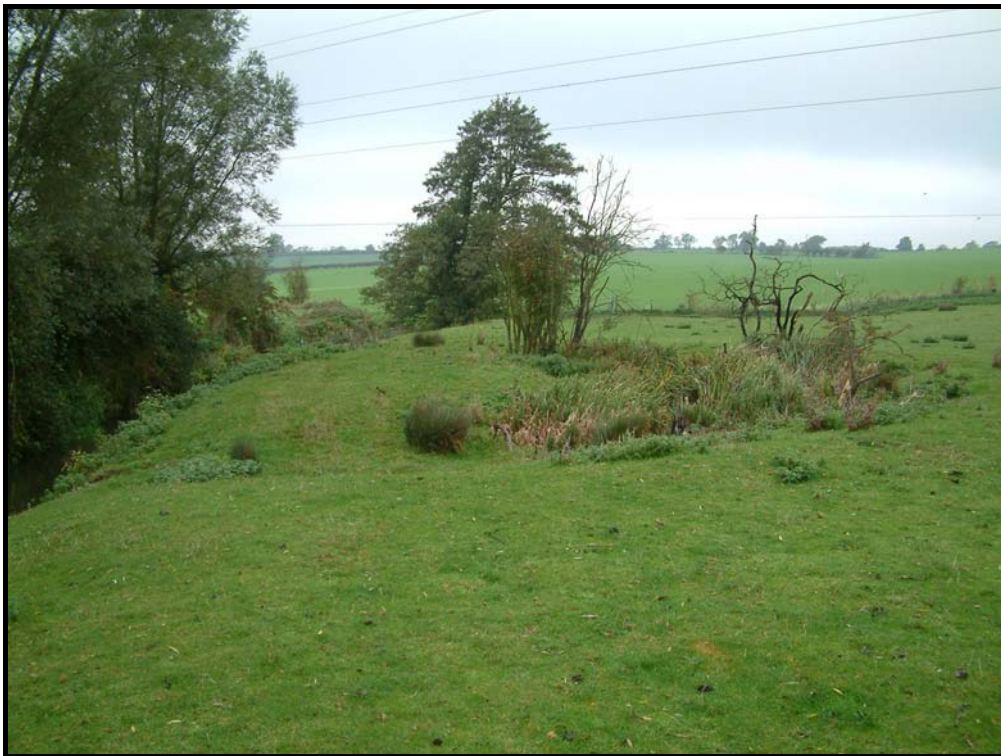
Plate 4 Harper's Brook looking north, showing the new channel and the made ground filling the old channel
