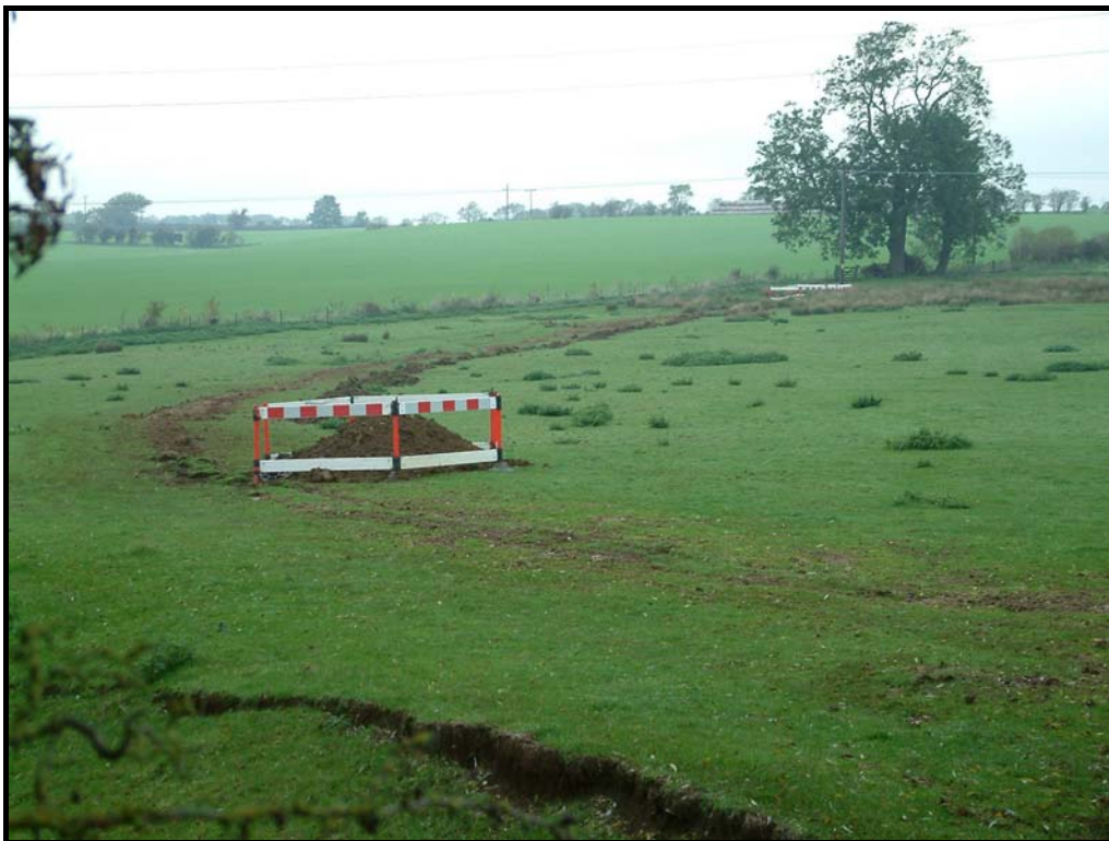
Plate 2 Henslow Meadow showing alignment of cable trench, looking north-east (Note erosion of made ground along edge of Harper's Brook in foreground)
