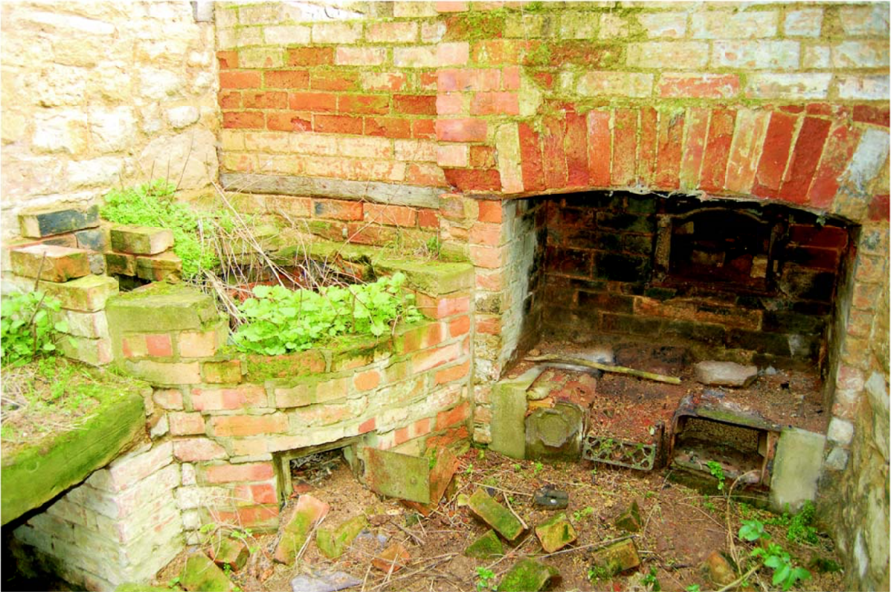
Plate 25: Water heater in north-east corner of Room 11.
