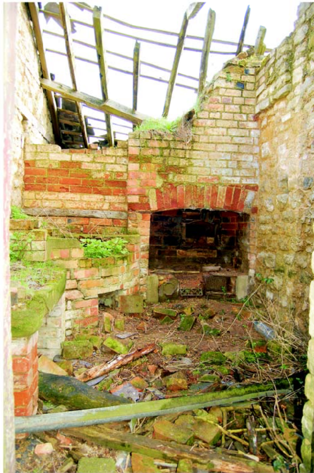
Plate 23: Stone sink, water heater, cast iron stove and bread oven in Room 11, looking east.
