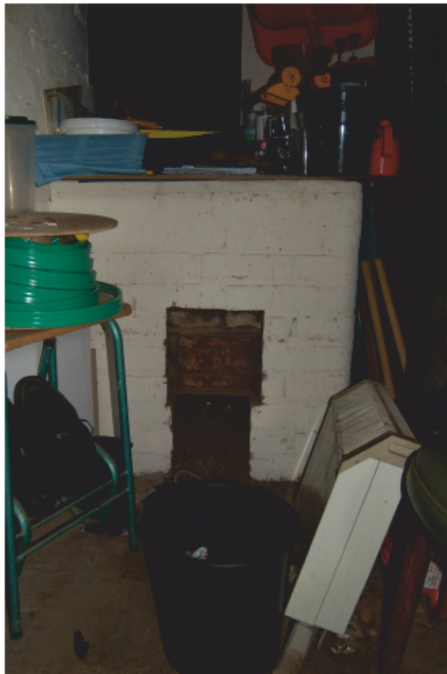
Plate 8: "Copper" water heater looking east.
