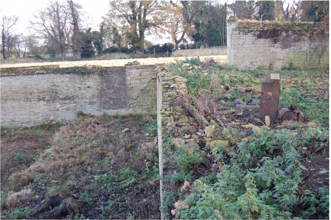
Plate 3: The west wall of the Walled Garden, the terrace within it (to the left) and the blocked doorway at the southern end of the terrace formerly leading to the Bowling Green beyond.
