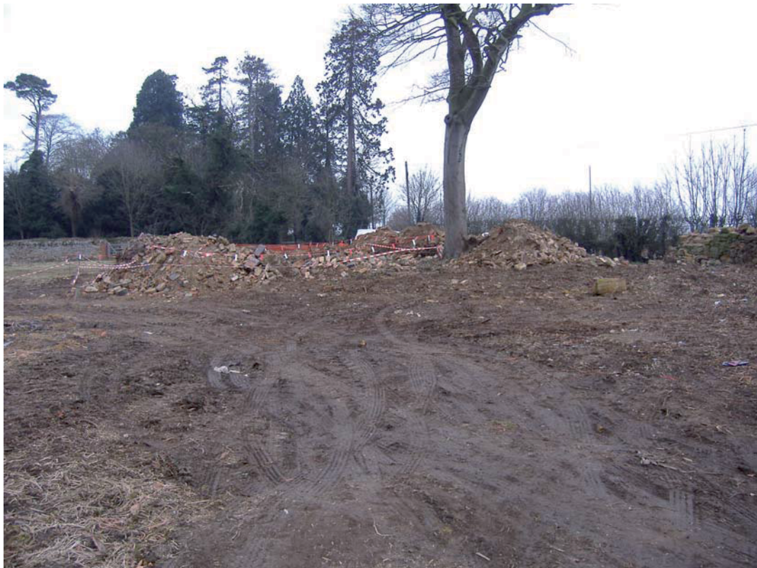
Plate 2: The area of the derelict buildings after demolition with the boundary wall in the background
