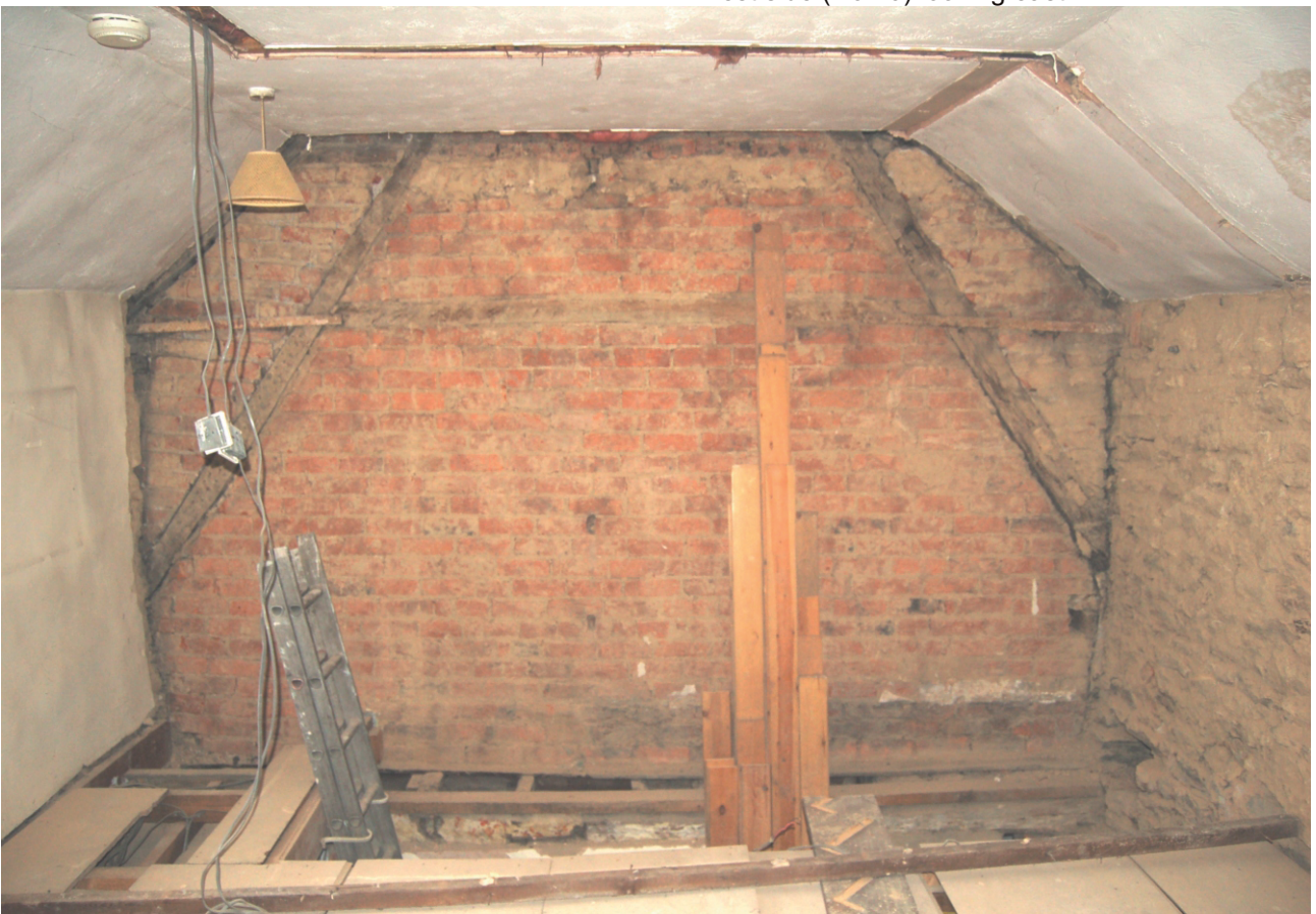
Plate 8 Dividing wall between cottages at first floor level showing original rafters and brick infill looking east from No 20
