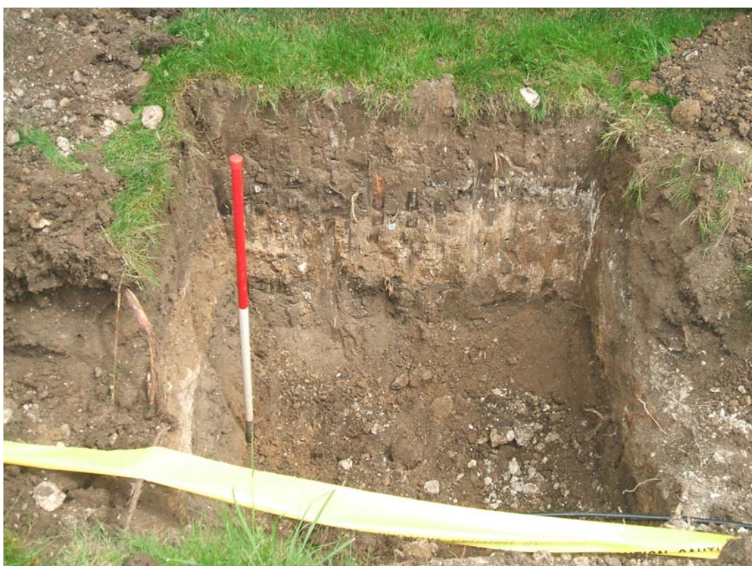
Plate 4: The soak-away pit
