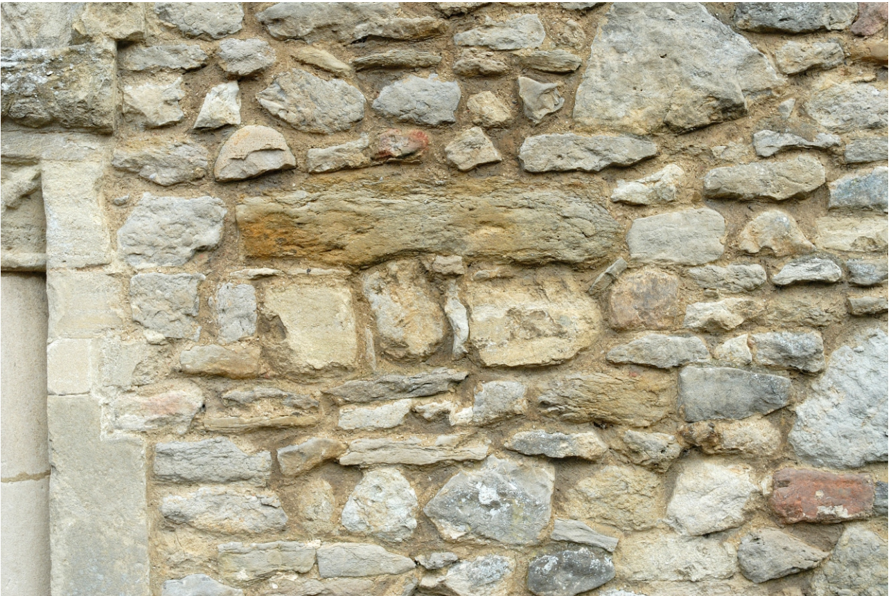
Fig 11: Blocked put-log hole
