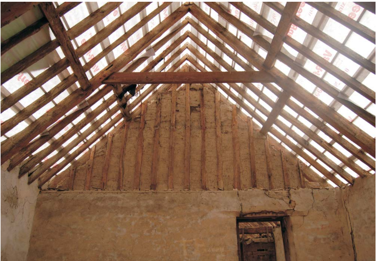
Plate 28: Internal cheek above eaves level infilled with stud and laths covered in plaster
