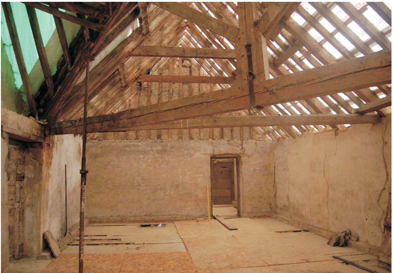
Plate 36: Dragon beam at junction of beam and post showing iron strap, Room 4
