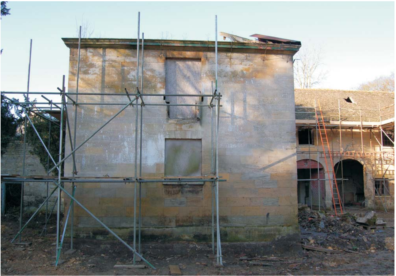
Plate 11: East facade of the south wing looking west, altered window at first floor
