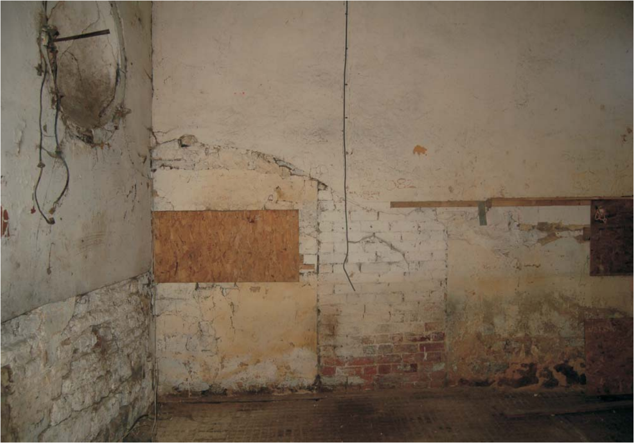
Plate 25: Blocked doorway and scar of stall, north wall of stable 2, looking north
