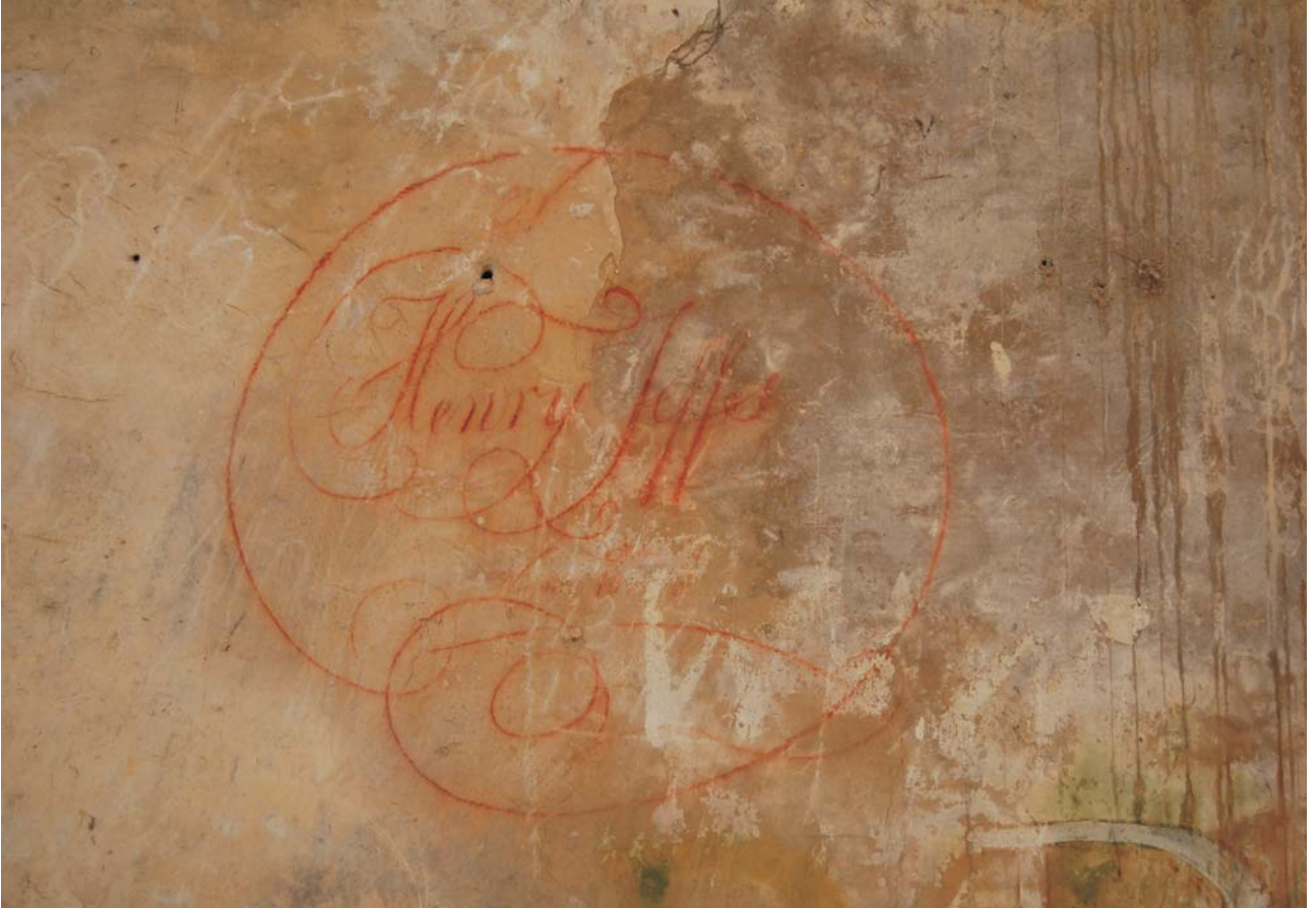
Plate 34: Red chalk graffiti on east wall of Room 3; Henry Jeffs
