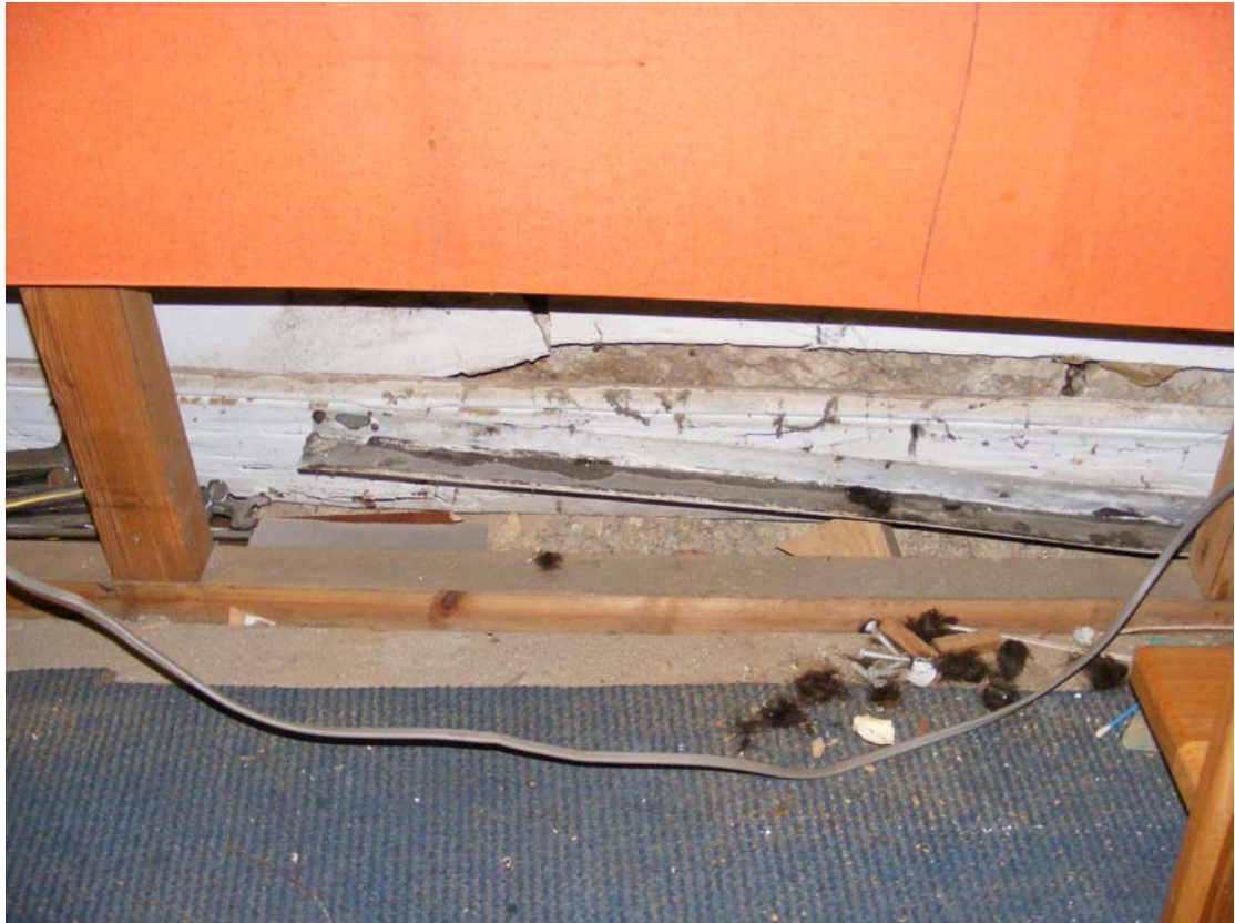
Fig 13: Obscured skirting in G4
