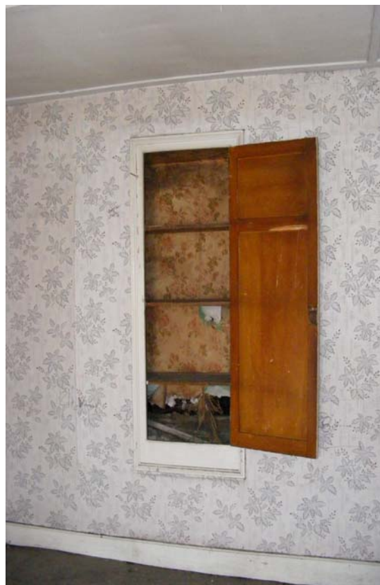
Fig 34: Cupboard in north wall of F5 – possibly a blocked doorway or window
