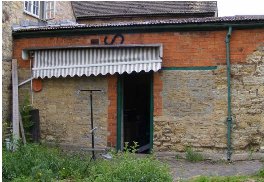
Fig 24: Brick eaves heightening of G5, viewed from the courtyard, note blockings also
