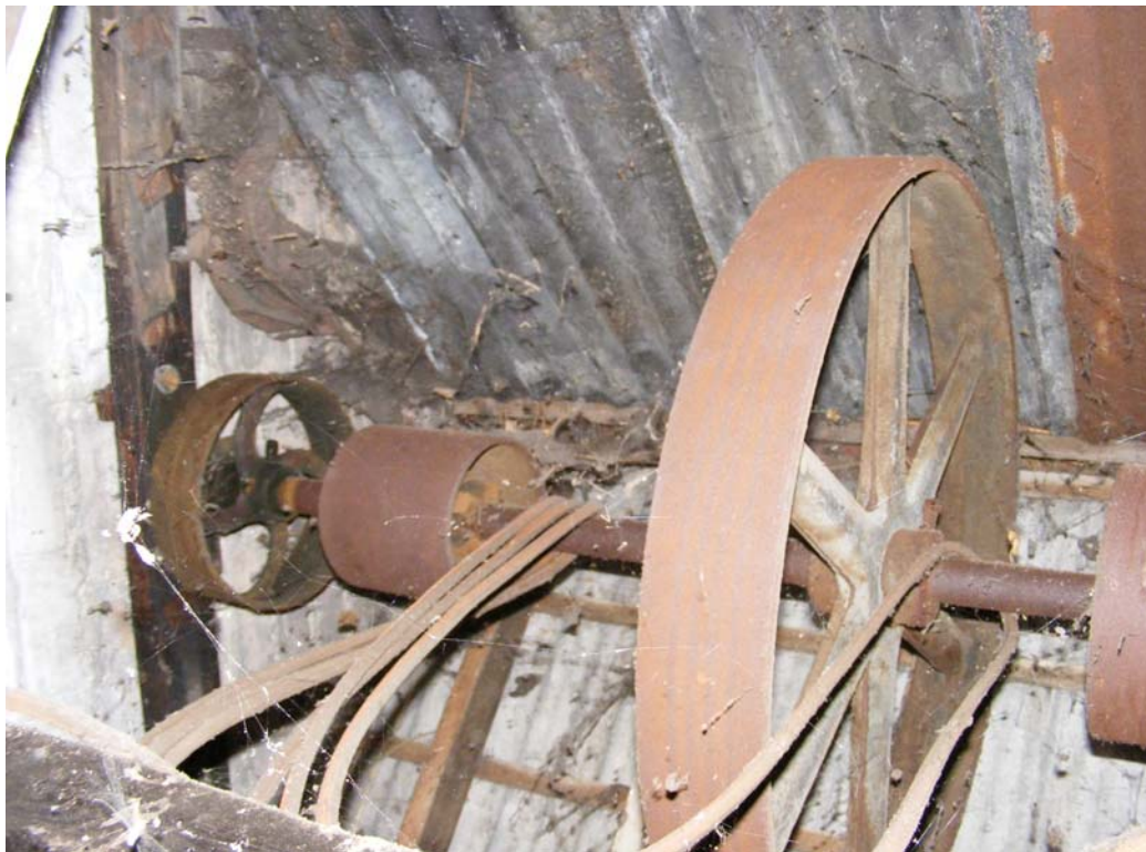
Fig 43: Pulleys and driveshaft above engine house/wc
