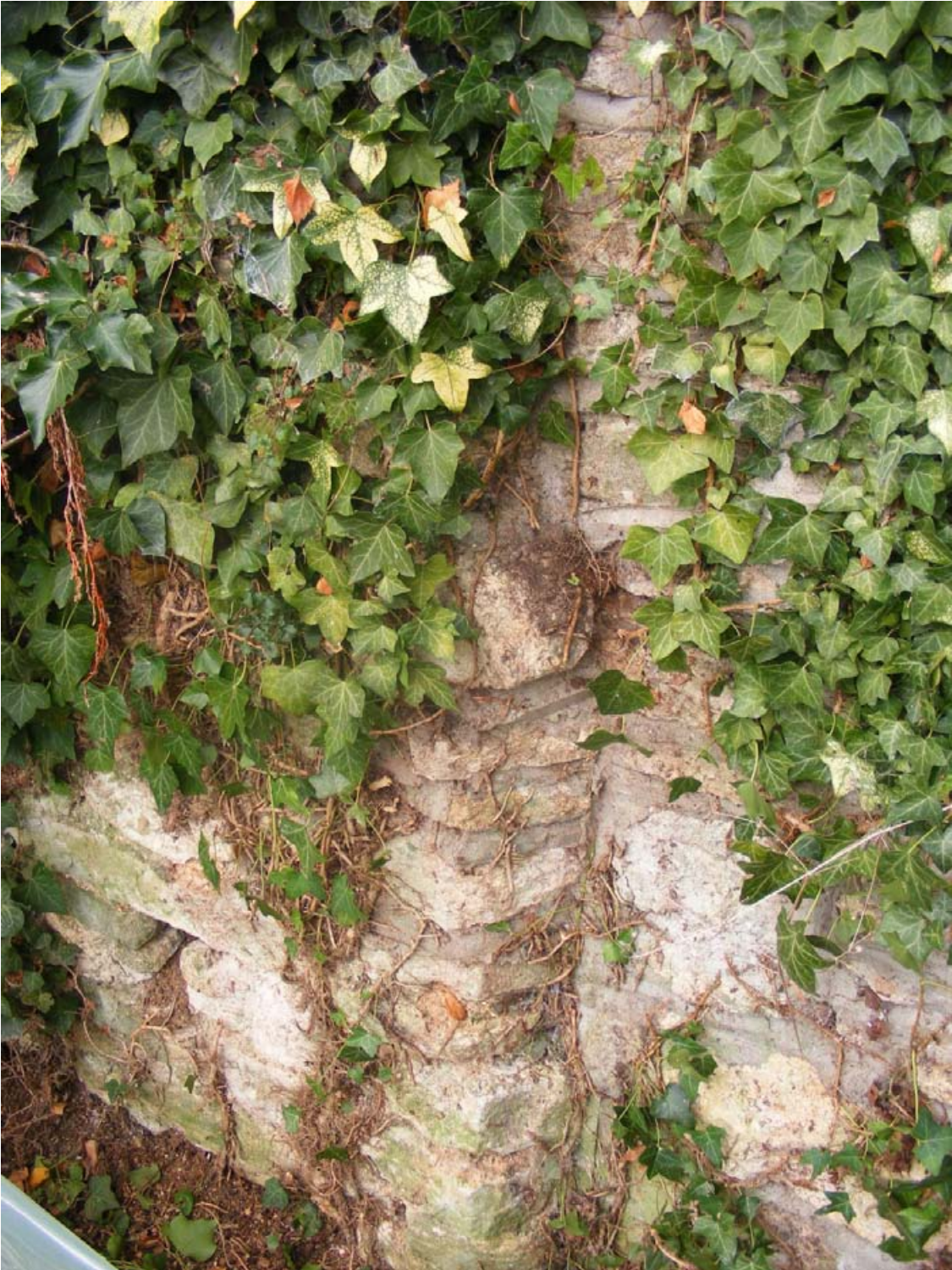
The eastern barn third bay and wall rebuild from the development area, looking north-west
