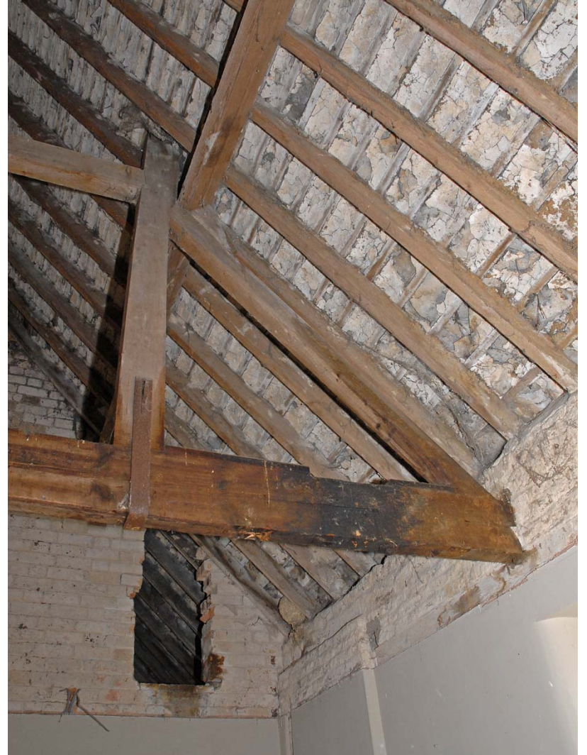
Fig 15: Room 2 truss detail showing oil staining
