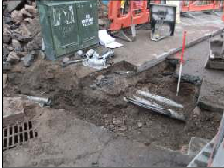
Plate 5: Connection Pit at the Western End of the Excavated Trench (facing south)
