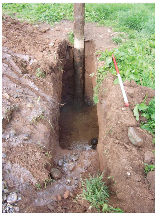
Plate 2: Excavated trench to the east of the existing electric pole (facing west)
