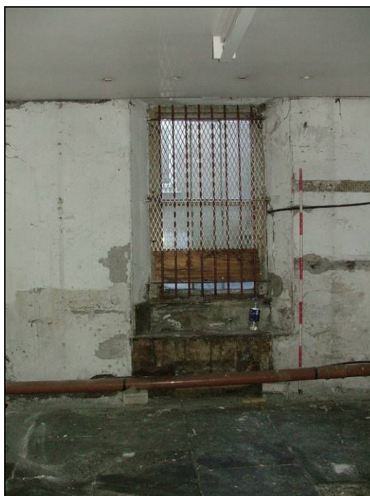
Plate 43: Detail of window with window seat and panelling below, ground floor, former kitchen (Scale = 2m)
