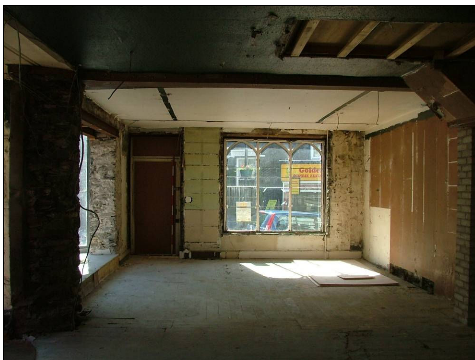
Plate 25: View looking east showing the interior of No. 2 Victoria Street, ground floor
