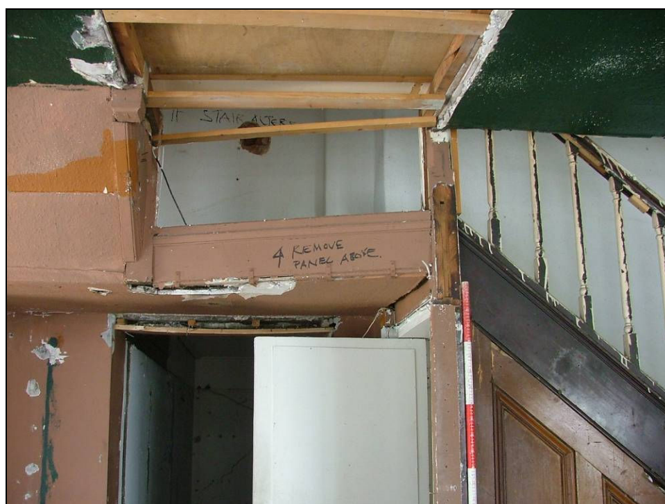
Plate 35: View looking south showing the possible former location of the stairs, ground floor of northern room
