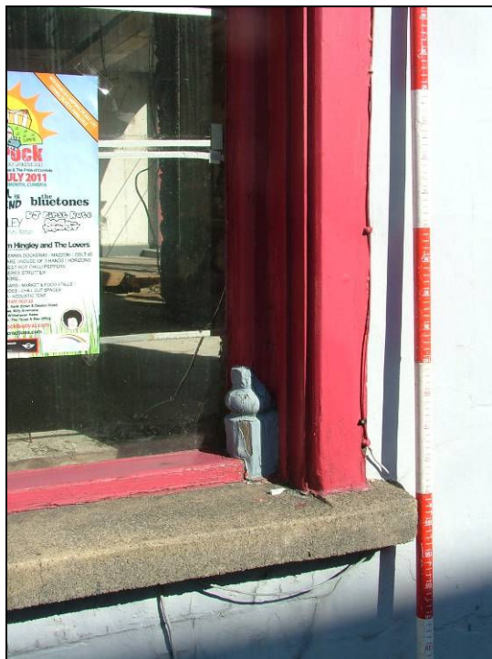
Plate 22: Detail of concrete sill and part of the ornamental timberwork of the window surround, east elevation
