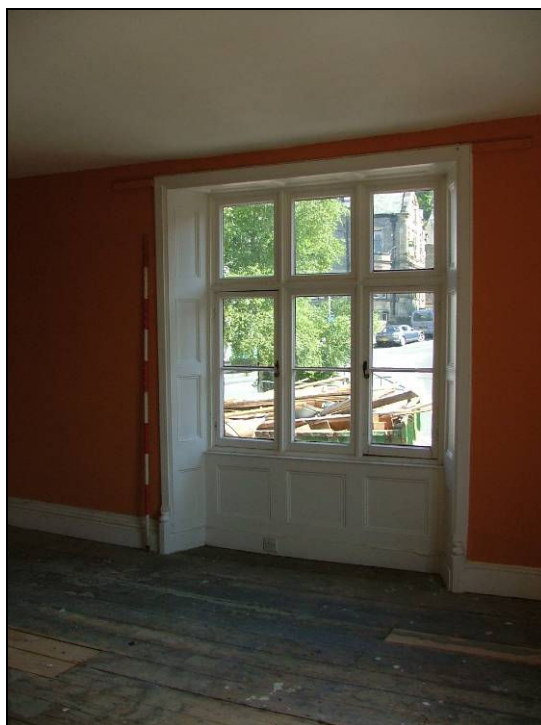
Plate 55: Detail of large window with panelled surround, north wall, first floor (Scale = 2m)
