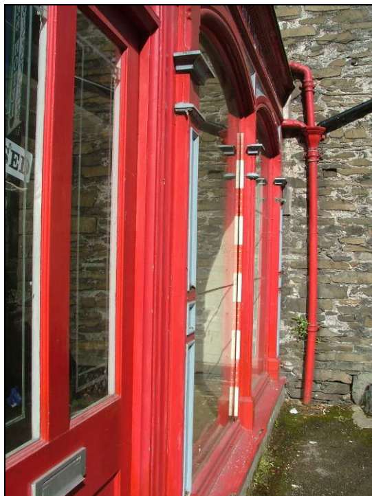
Plate 14: View looking west showing the timberwork of the shop front, north elevation of No. 2 Victoria Street (Scale = 2m)
