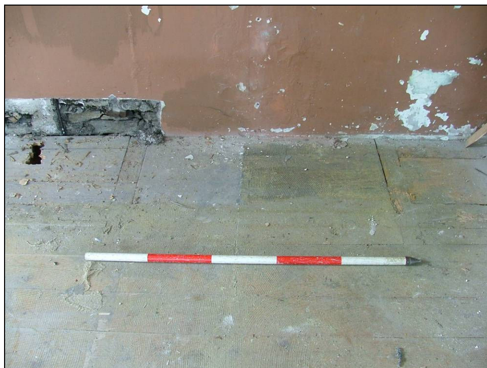
Plate 33: Evidence for a former fireplace, east side of ground floor room (Scale = 1m)
