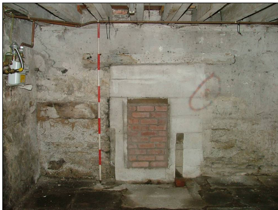
Plate 51: Possible blocked opening or location of a former heating system, cellar (Scale = 2m)
