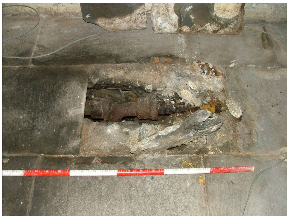
Plate 49: Exposed pipework beneath the floor of the cellar
