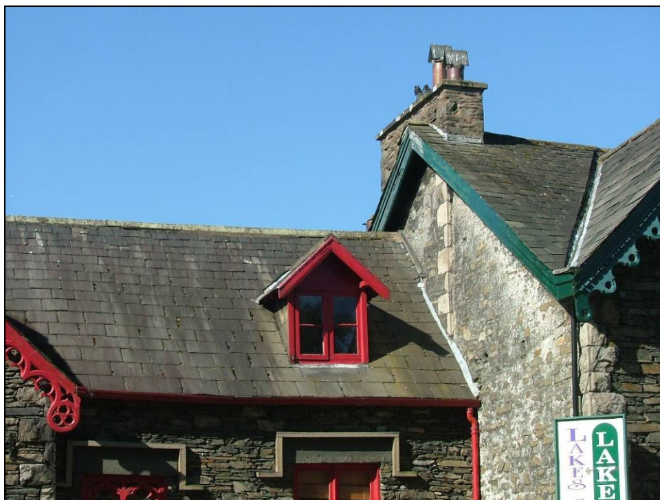
Plate 10: West side of the roof of No. 2 Victoria Street where it butts up against No. 1 High Street
