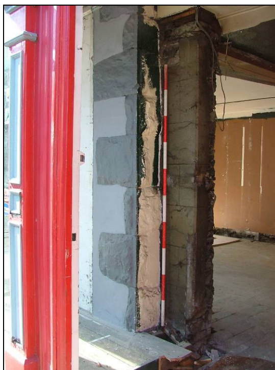
Plate 29: Detail of quoins of gabled projection as seen from the main entrance (Scale = 2m)
