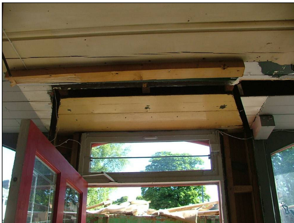
Plate 28: Evidence of former recessed doorway in ceiling of projecting shop front, north elevation of property
