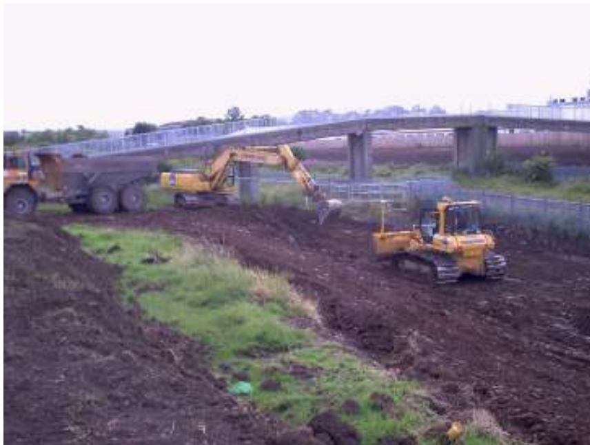
Plate 11: Contaminated soil strip to the east of the rail line, southern end
