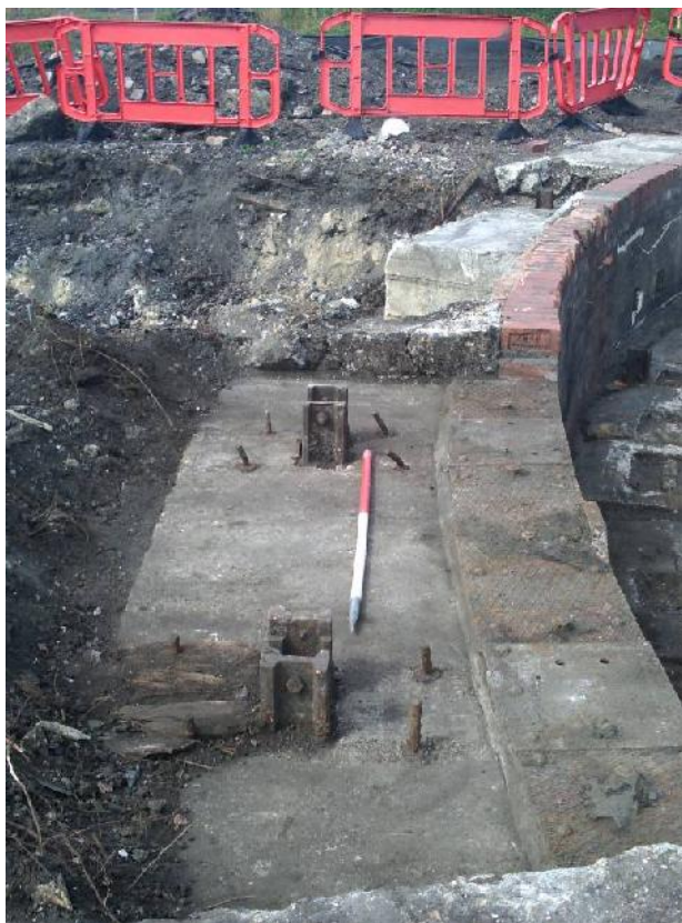
Plate 48: Fitting 4211. Facing West.
