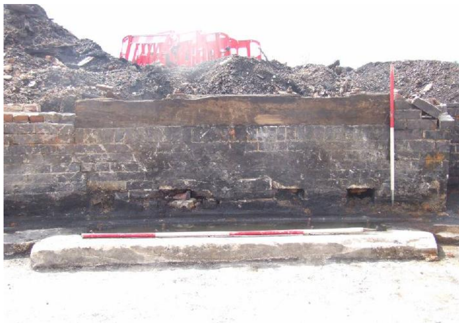
Plate 44: Interior of Turntable 1, Showing Beam 2209, Openings 2210 and (foreground) Concrete Pad 2211. Facing South-east.
