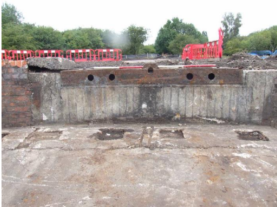
Plate 49: Fitting 4210. Facing North.
