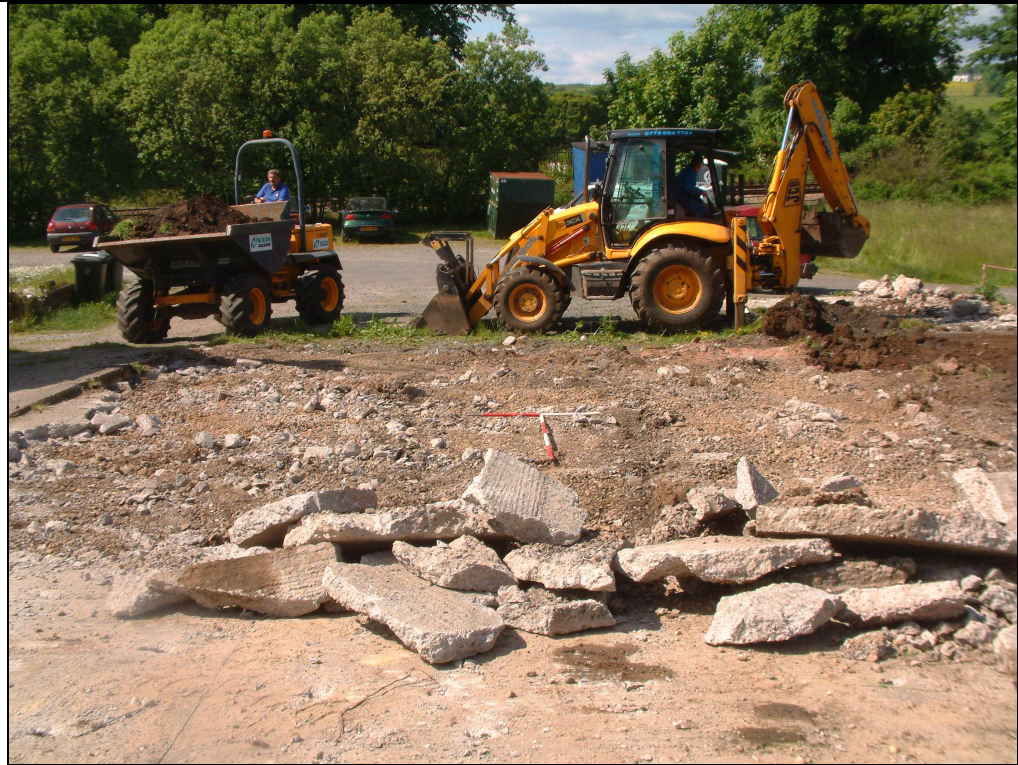
Plate 2: Area of concrete partly broken up and lifted to reveal sub-base on day two
