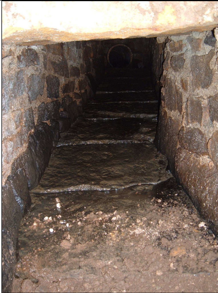
Plate 10: Stone lined culvert encountered on day five during the excavation of Trench Four
