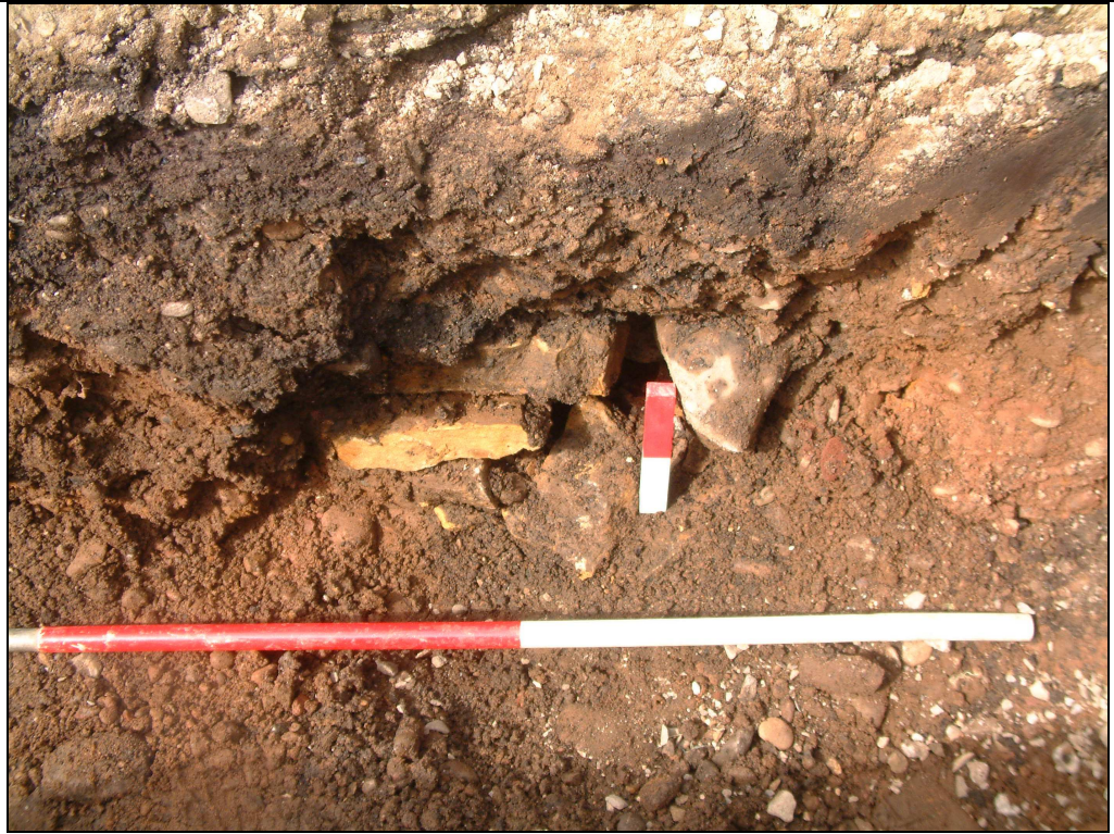
Plate 5: Stone drain/culvert observed in east facing section of western edge of Trench Two on day three
