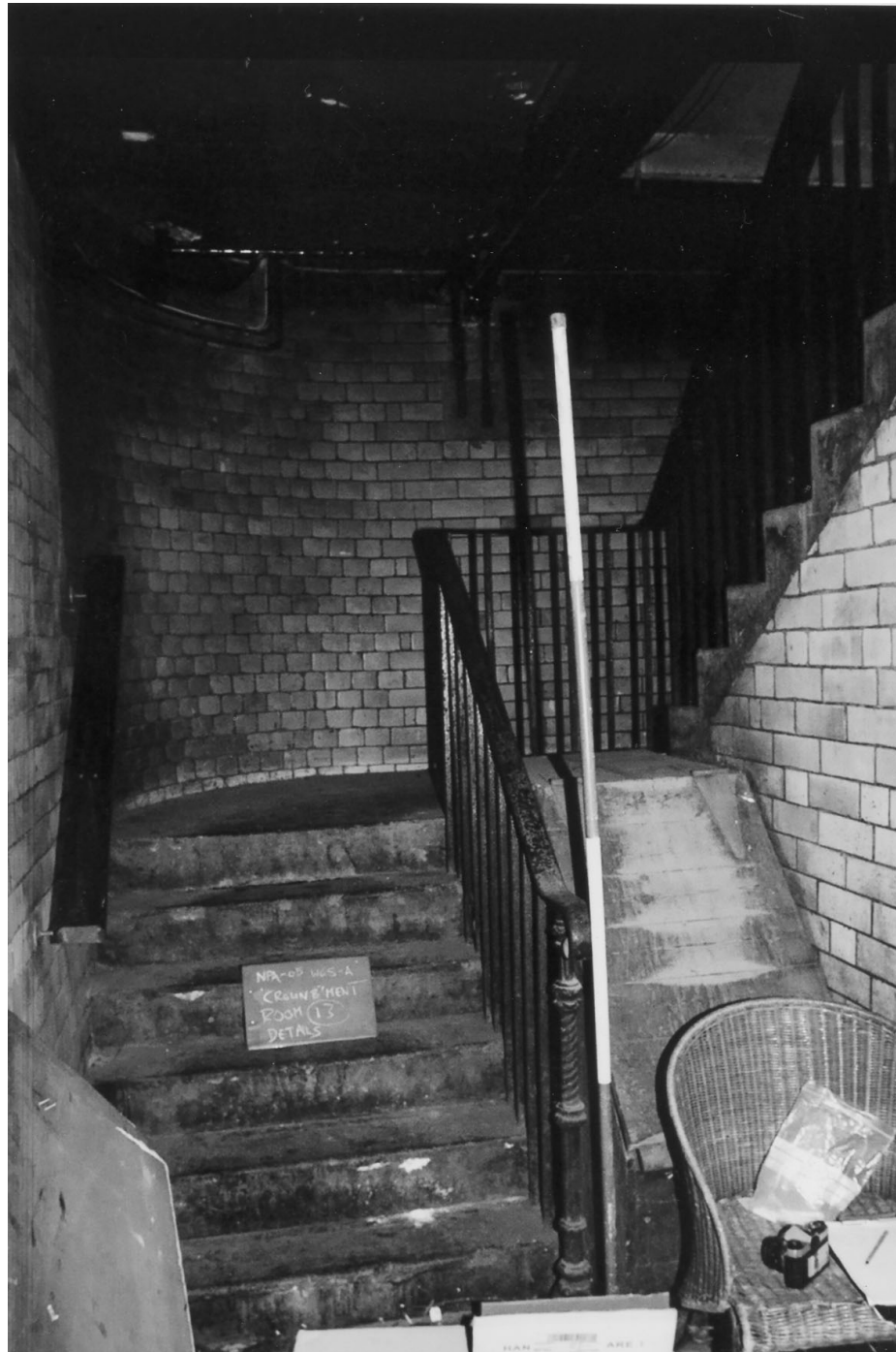
Plate 33: 33 High Bridge. Basement Room C13, looking south. Main stairwell for shops and offices of 1901.
