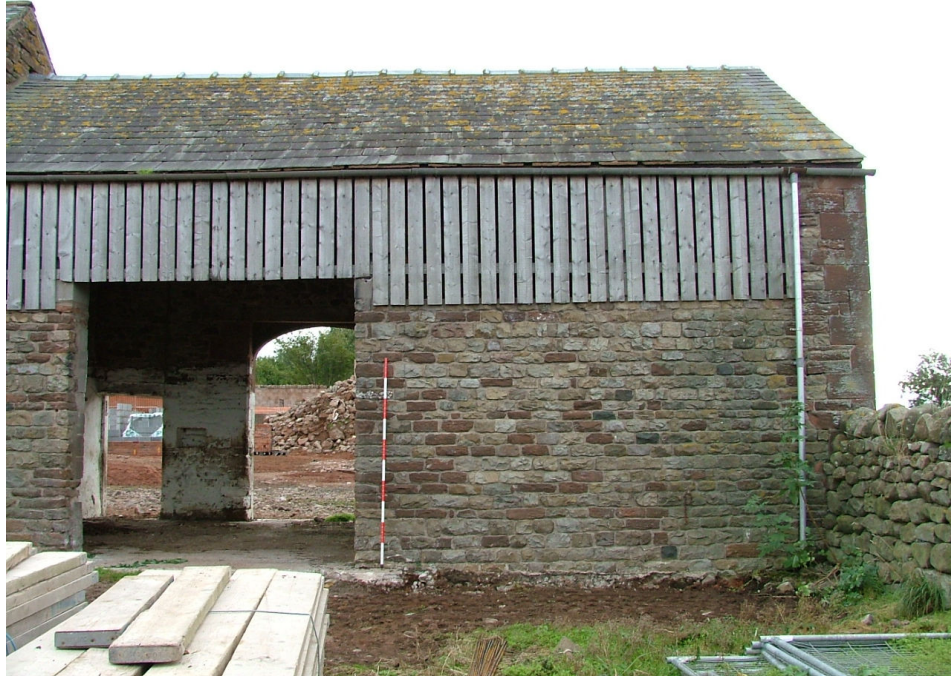
Plate 8 – Northern elevation of the cart shed showing stonework hiding a block wall
