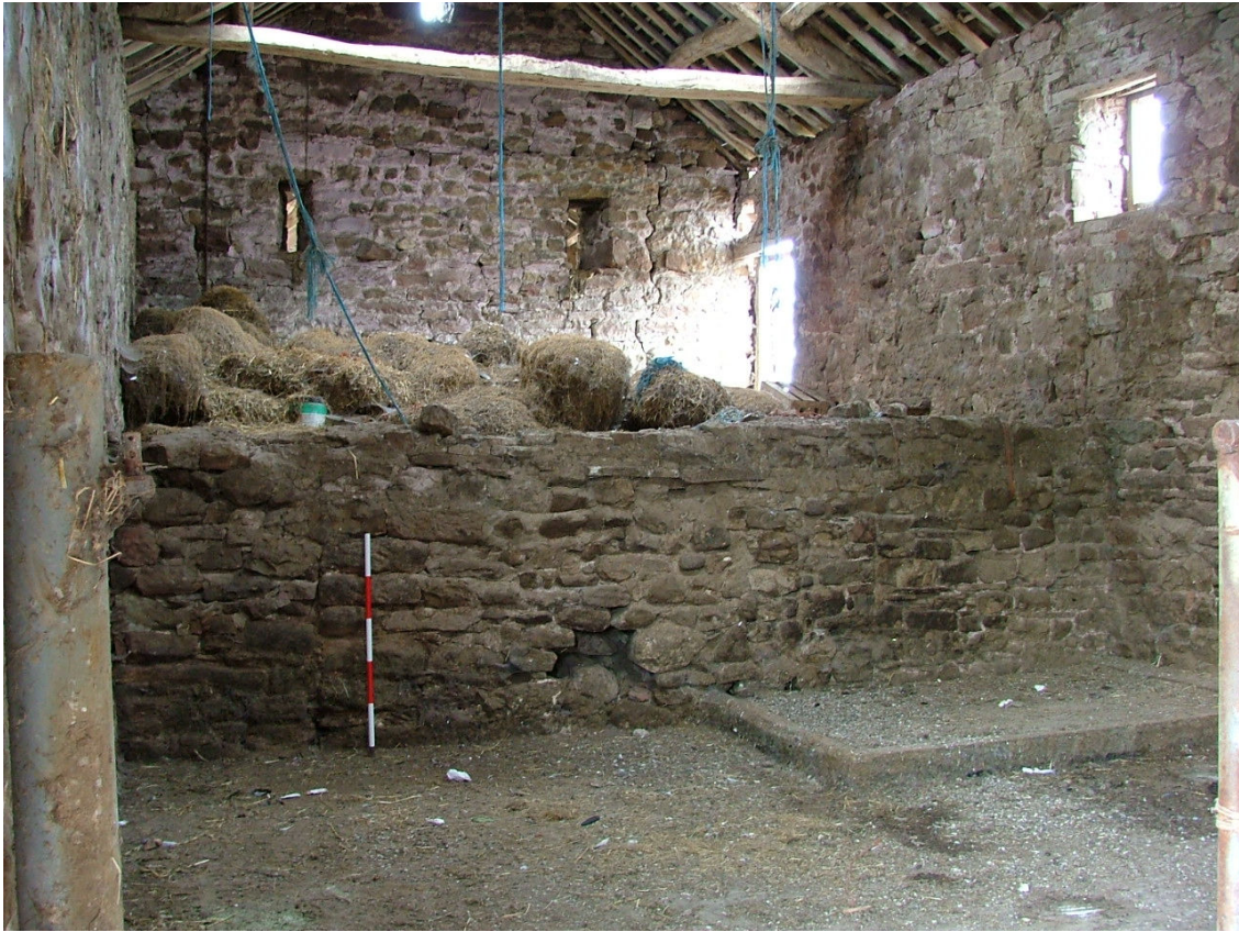
Plate 12 – View of the hayloft above the western byre as seen from the threshing area
