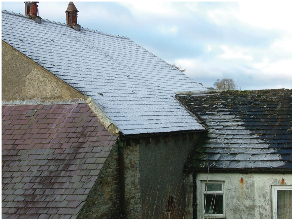
Plate 10 – Join of the roofs of the main chapel, the school room (left) and the adjoining cottage (right)
