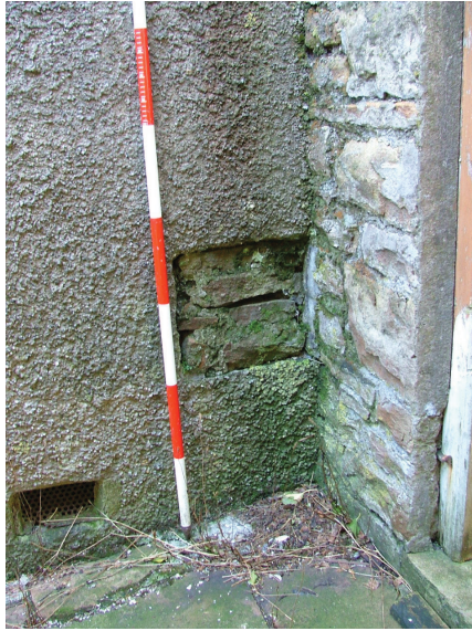
Plate 13 – Blocked hole, south-east elevation
