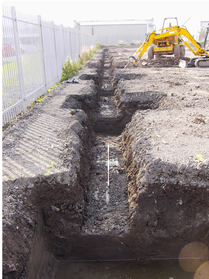
Plate 3. The excavation of the southern arm of Units 4A-4B, 5 and 6, looking west.
