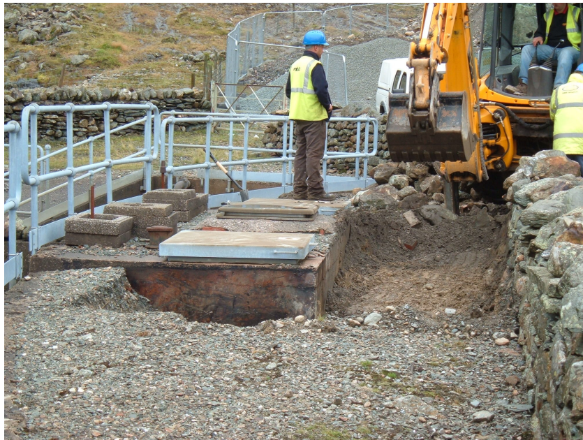
Plate 6: Photograph Showing the C-Shaped trench for ducts to the west of the existing Water Treatment Works Building
