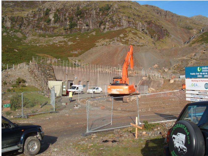
Plate 3: The Paddy End Water Treatment Works site after Ground Works were completed (September 2006)
