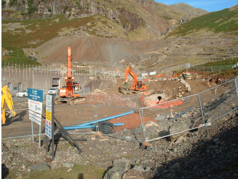
Plate 5: Location of the main works, with the new road on the right, stream at the centre and building extension due to be inserted by the furthest machine at the centre
