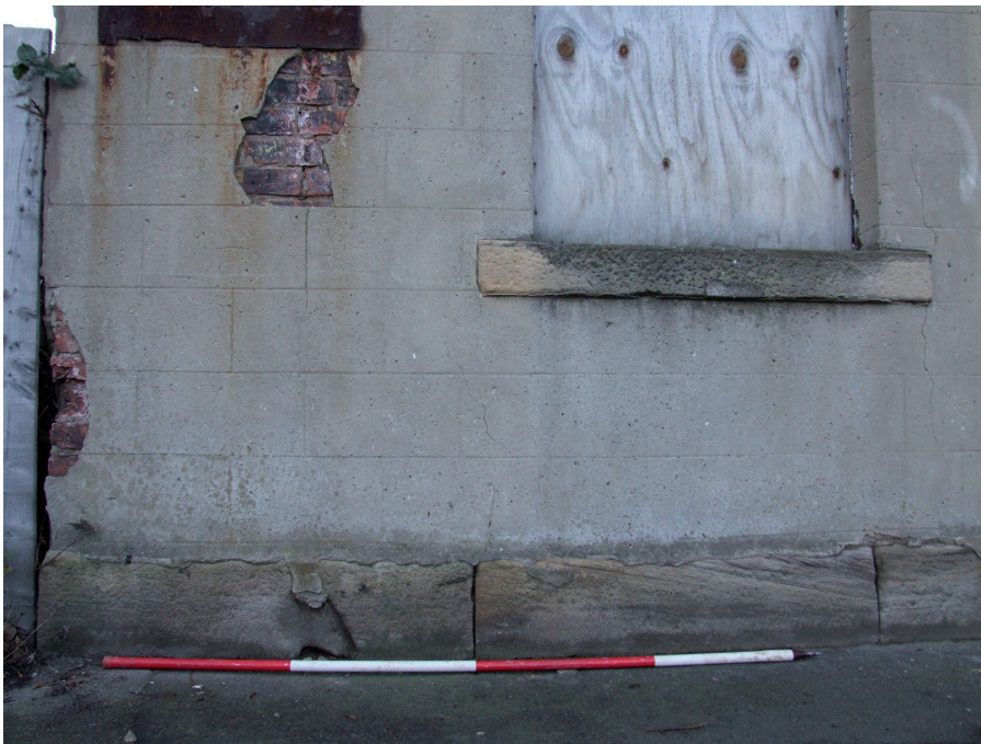
16.) View of 'A1', sandstone foundation course, window corbel, and Victorian cement render with exposed underlying brickwork.
