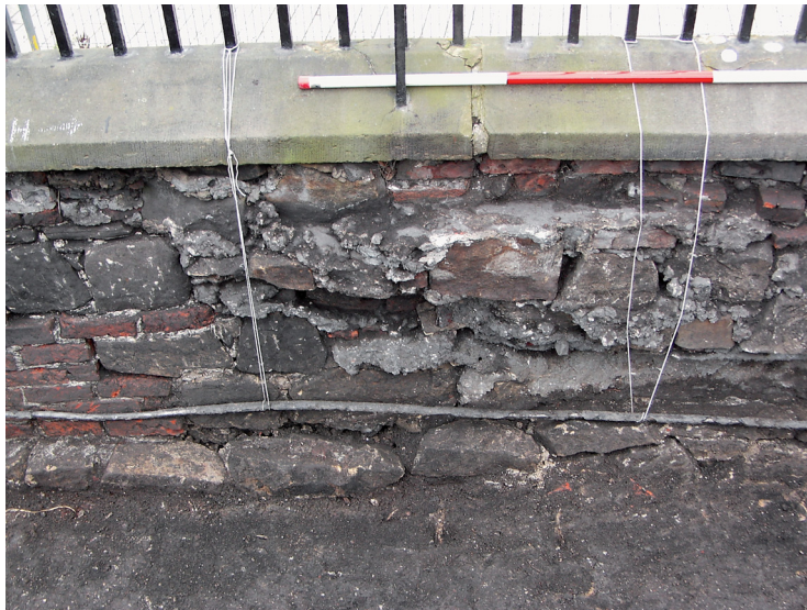
Plate 13. View of excavated trench showing the poor concrete and stone repair on the weakest section of the wall. The service cable can be seen left in situ and supported on the railings.
