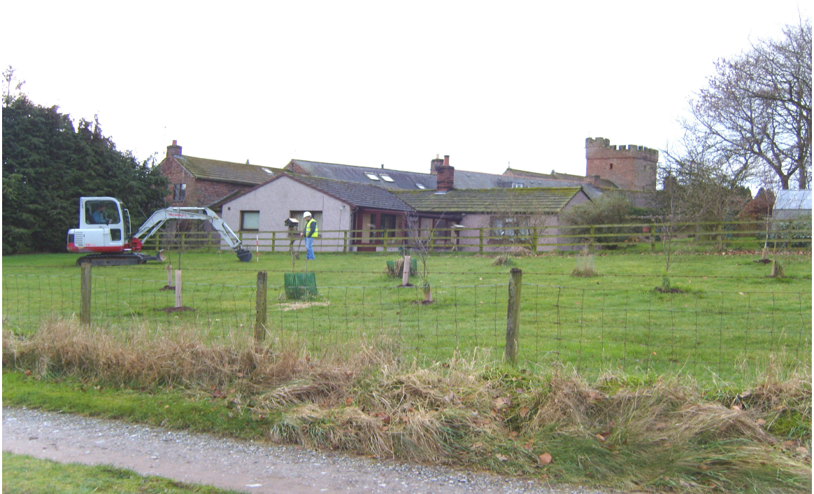
Plate 6: Trench 1 under excavation, showing St Cuthbert's Church in the background, facing west
