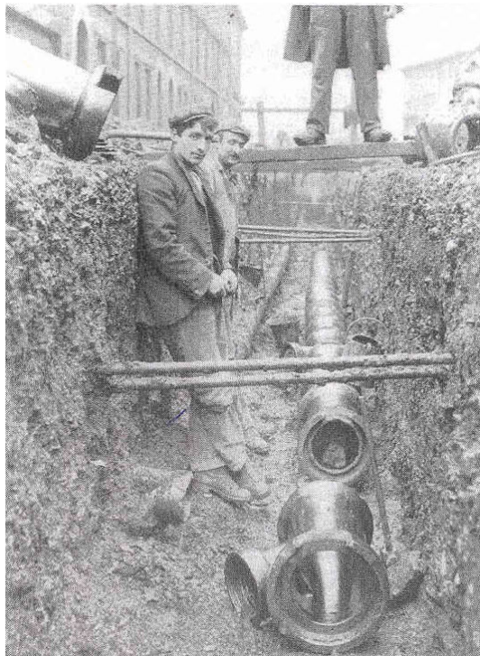
Plate 1: Laying the sewer pipes in Ann Street at the end of the 19 th century. (From Bingham, 1995).
