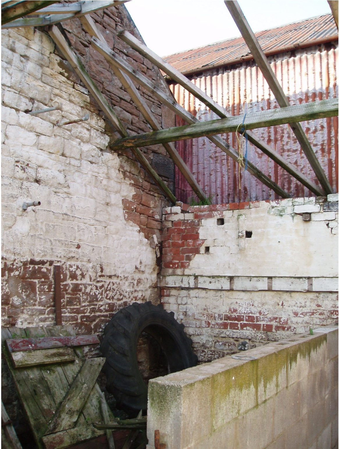
Plate 7: Interior of one of the buildings showing brick partition walls and timber roofing frame, with a modern addition of a corrugated iron barn behind.
