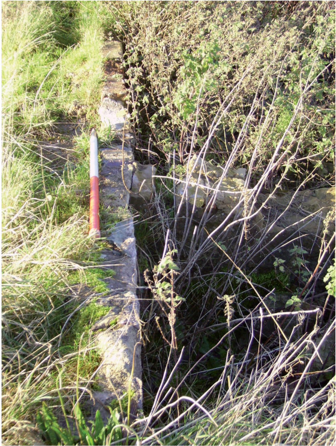
Plate 3: section of partially buried wall towards southern extent of scrubland, facing west
