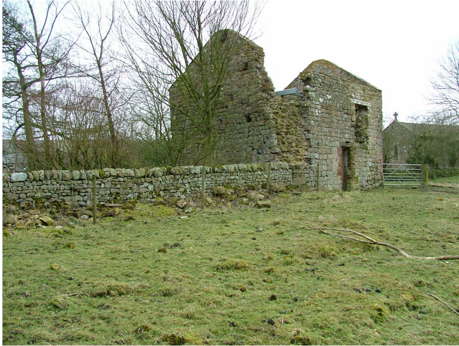
Plate 8 – Collapsed north-east corner of the bastle house, with rubble masonry piled against the garden wall
