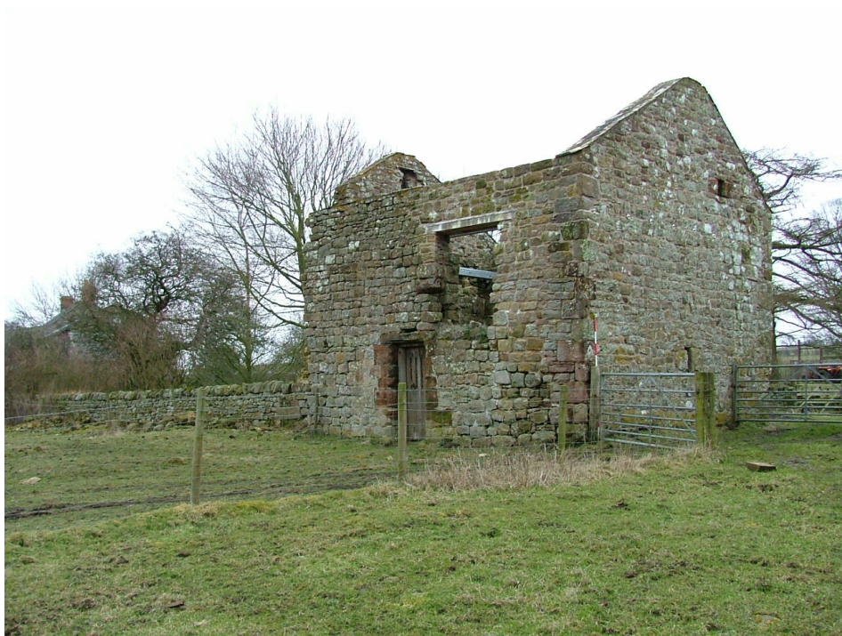
Plate 7 – Northern elevation of bastle house showing dry stone wall to east which forms part of the garden boundary wall
