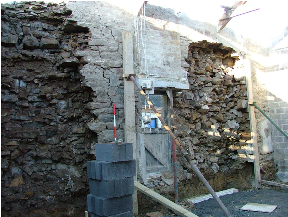
Plate 10 – Sections of the collapsed west wall
