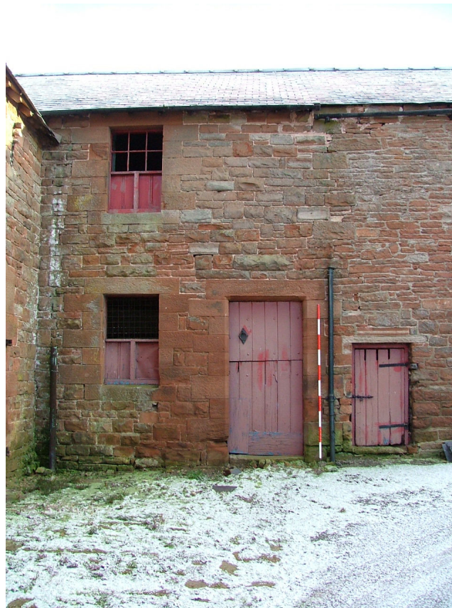
Plate 9 – Location of construction break, masonry to left of ranging pole is coursed and consists of large blocks, to the right the masonry is thinner and is roughly coursed and dressed
