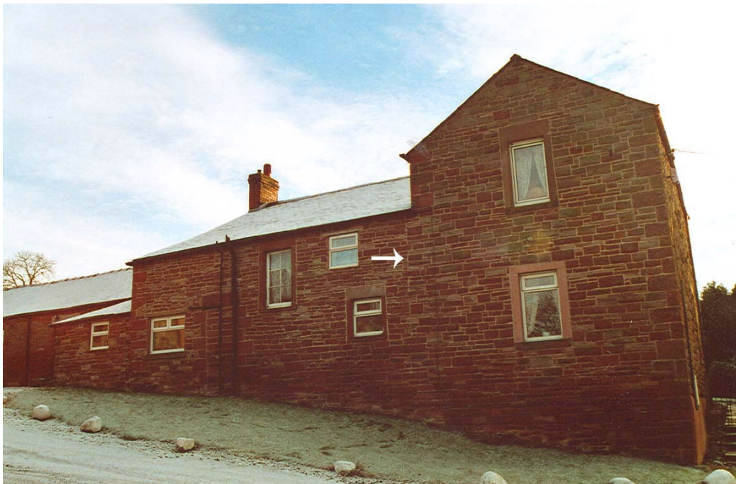
Plate 24 – Northern elevation of farmhouse, white arrow shows location of construction break
