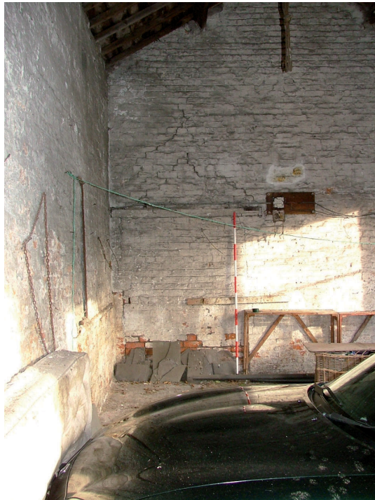
Plate 11 – Larger of the two blocked doorways, central interior dividing wall (looking north)
