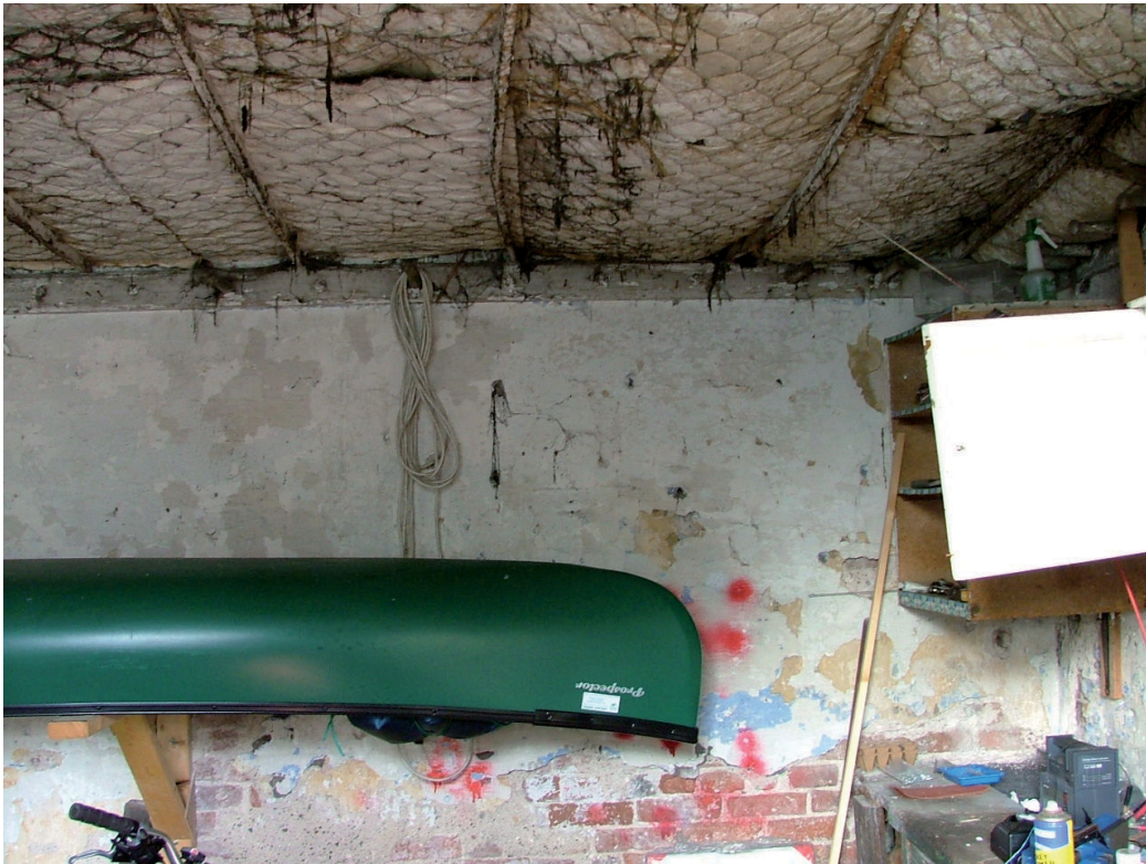
Plate 17 – Chicken wire and straw ceiling and wooden rails with pegs, northernmost room
