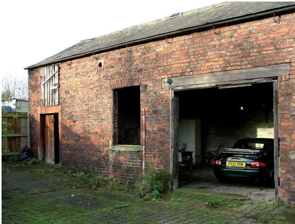
Plate 3 – Southern end of the east elevation, a change in brickwork can be observed to the right of the large doorway suggesting the opening was enlarged slightly
