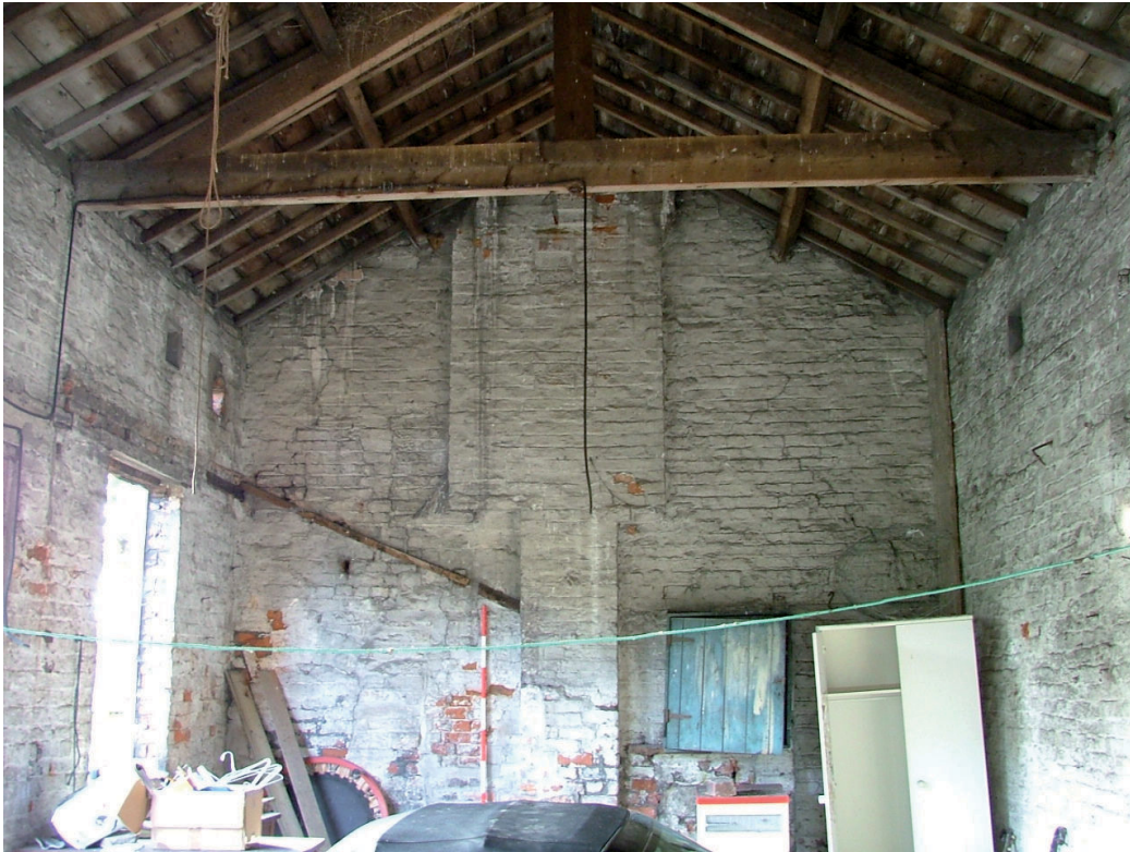
Plate 10 – Southern end of building, Blocked window visible to the left of photograph, blocked hatch(?) visible below blue cupboard and blocked doorway is behind the white wardrobe
