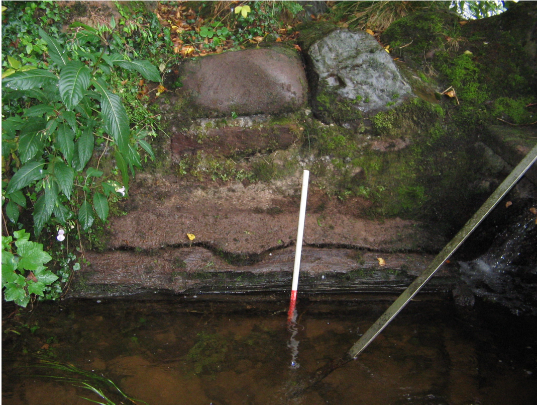
PLATE 15: CANALISED BREACH OF NORTHERN EYOT, LOOKING SOUTH
