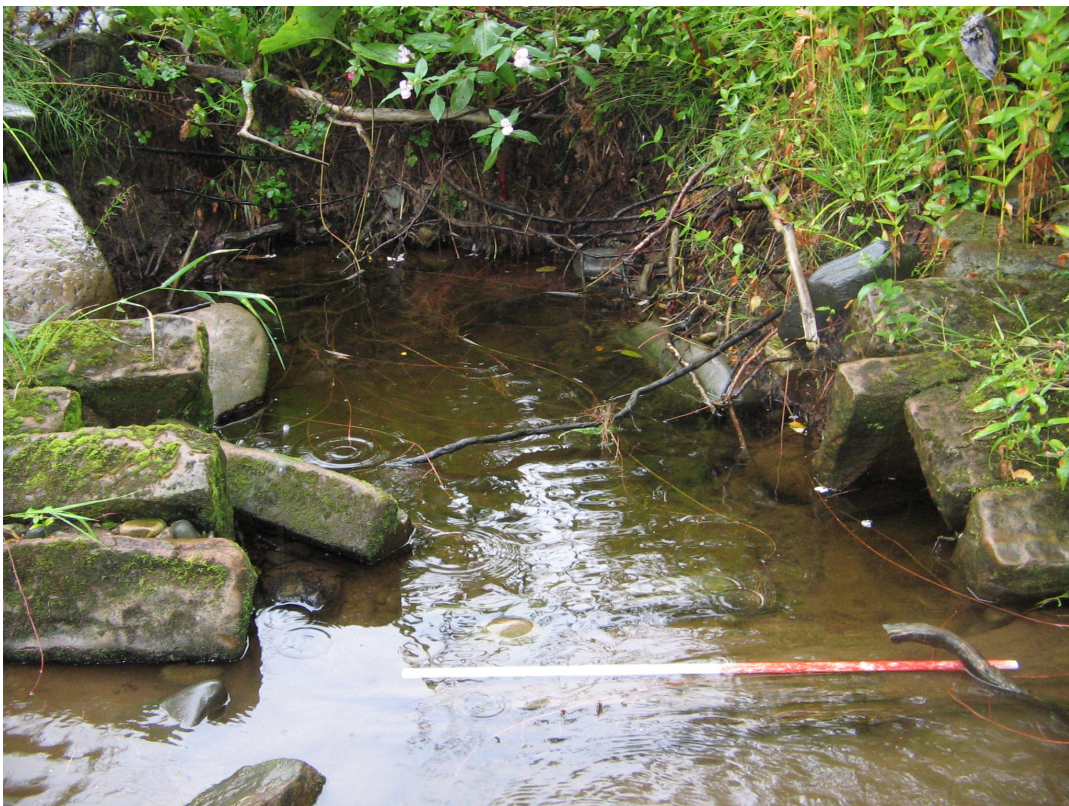
PLATE 16: DAMAGE TO STONWORK OF NORTHERN EYOT, LOOKING WEST
