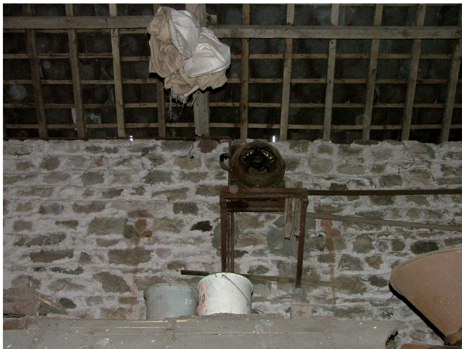
Plate 26 – Electric motor located above thresher in Building 4
