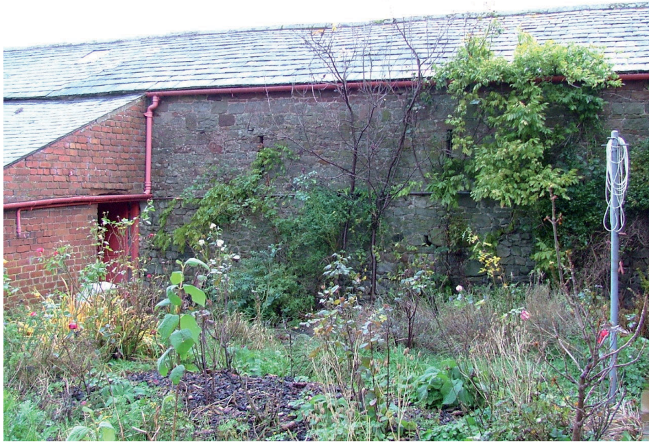
Plate 16 – Part of the southern elevation of Building 3, with a section of Building 6 visible to the left
