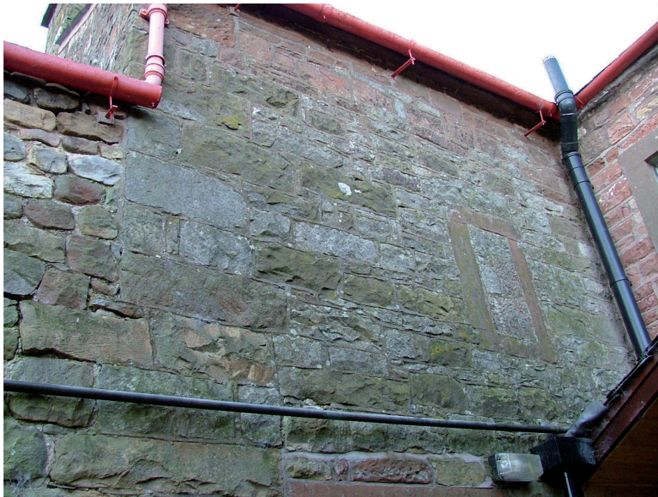
Plate 36 – West elevation of farmhouse showing different construction phases between the house and Building 1 (to the left), also shows a former window
