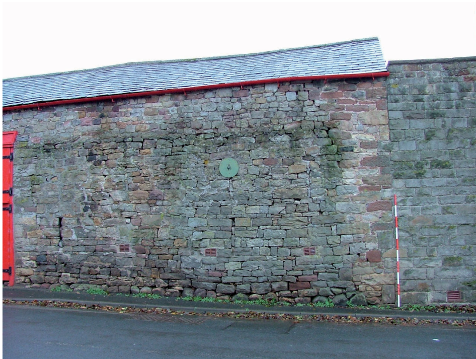
Plate 3 – Construction break between the two buildings that make up Range A (east facing elevation)
