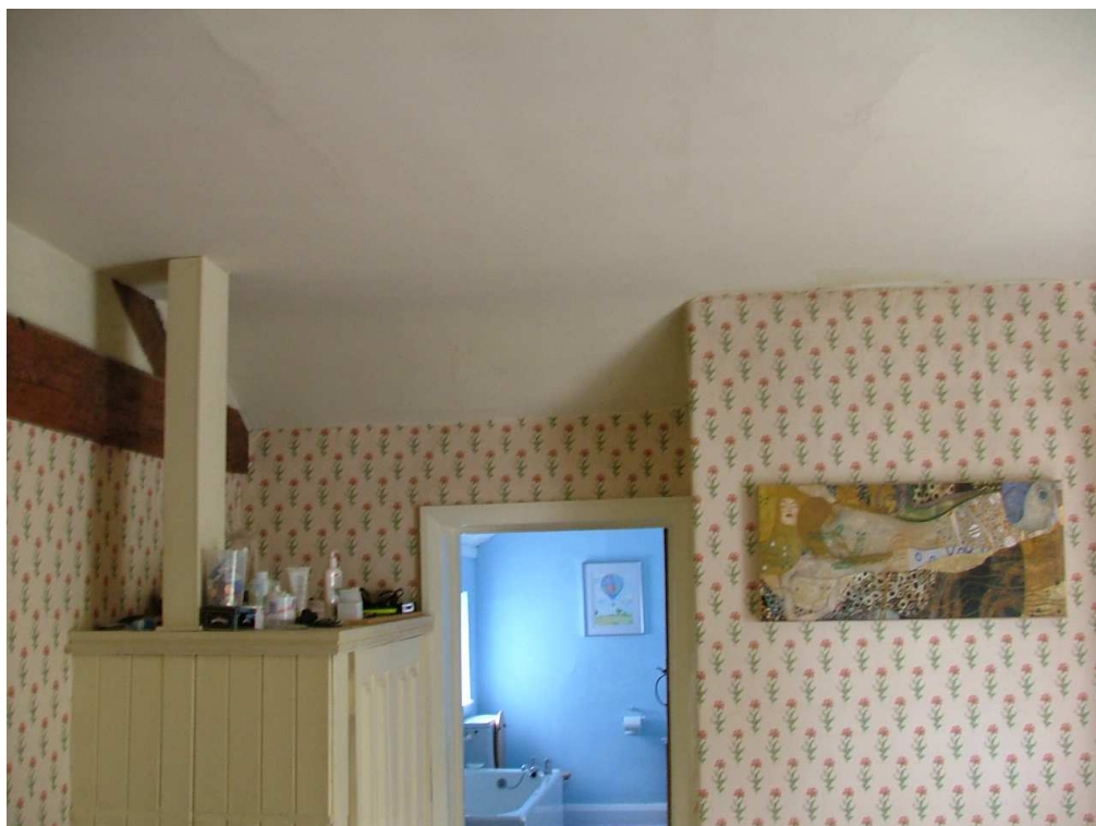
Plate 37 – Bedroom over the present kitchen showing exposed roof truss to left and curved ceiling (view looking west into the first floor of north-west extension)
