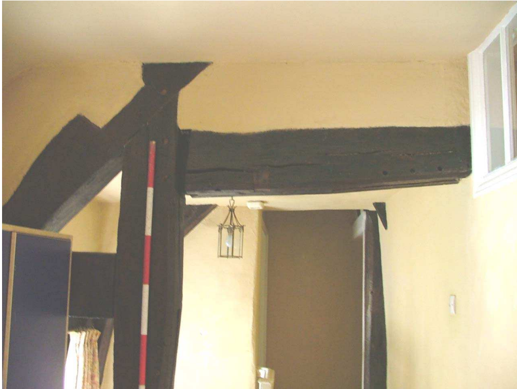
Plate 28 – Exposed timbers of former roof structure, first floor landing (Scale is in 20cm graduations)
