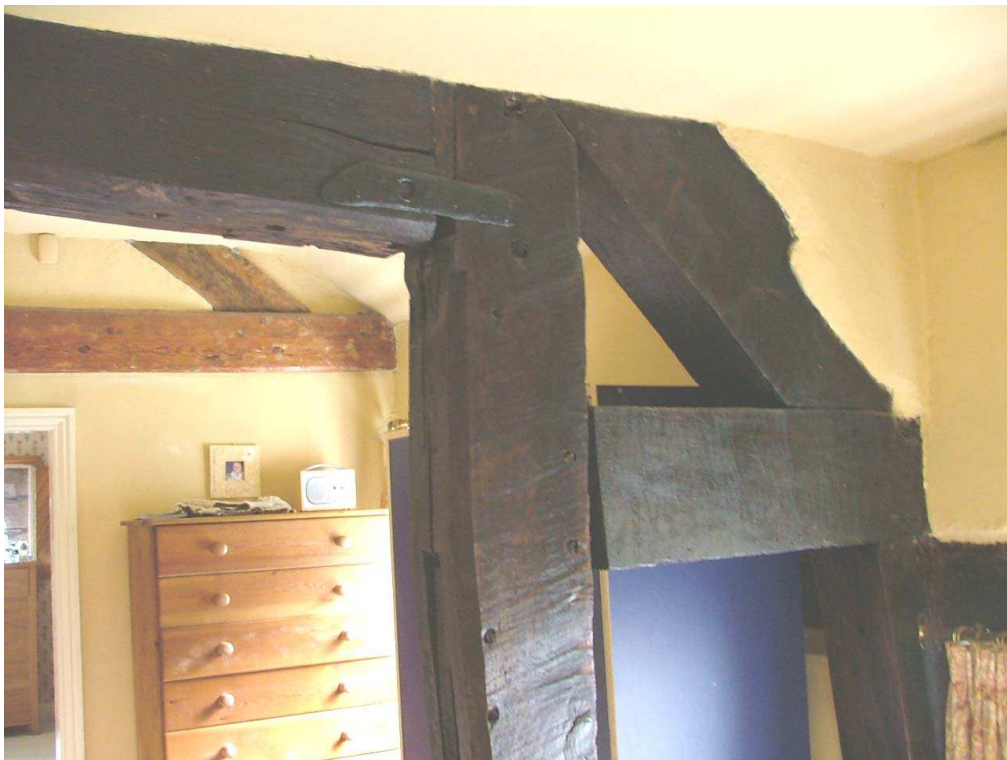
Plate 29 – Exposed timbers for former roof structure showing redundant peg holes and mortice
