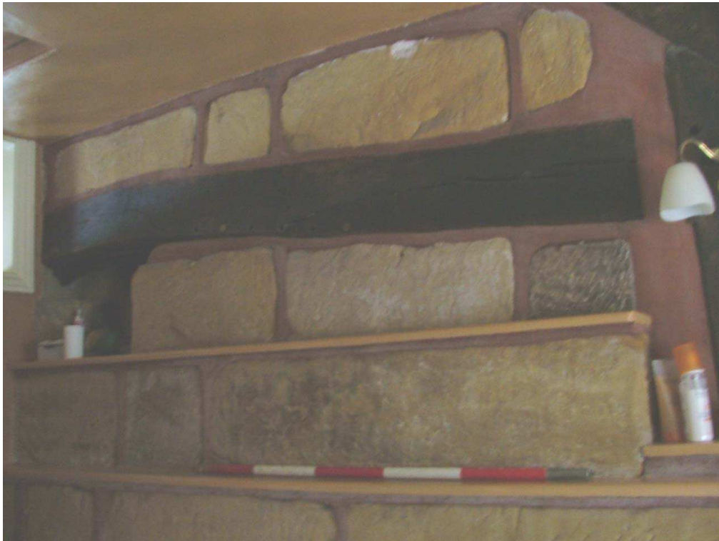
Plate 30 – Stonework of top of chimney stack built around pre-existing roof truss (Scale = 1m)
