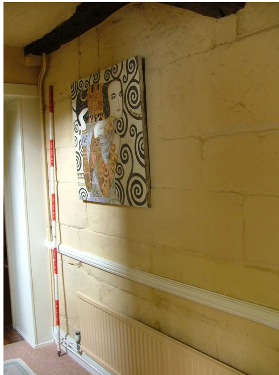
Plate 19 – Internal wall defining the west side of the hallway, constructed from large rectangular blocks of masonry (Scale = 2m)
