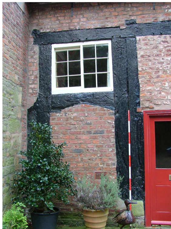
Plate 3 – Original doorway in east elevation showing depressed arch lintel, window above and projecting wooden pegs (Scale = 2m)
