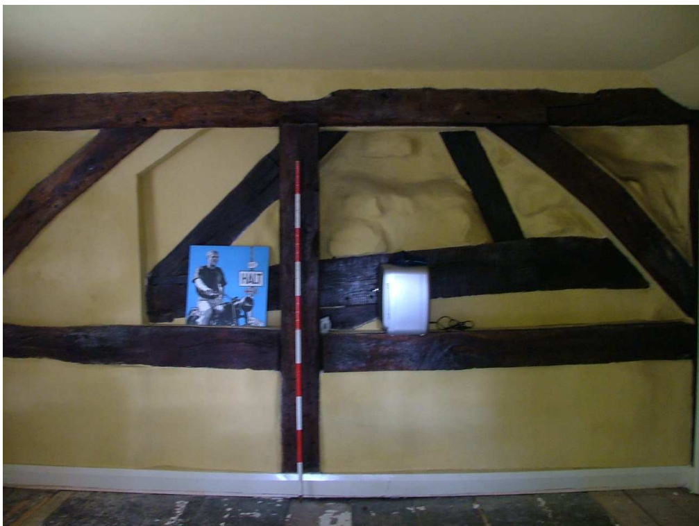
Plate 33 – Two separate phases of framing, north wall of bedroom in cross-wing. The truss behind appears to belong to the earlier hall (Scale = 2m)
