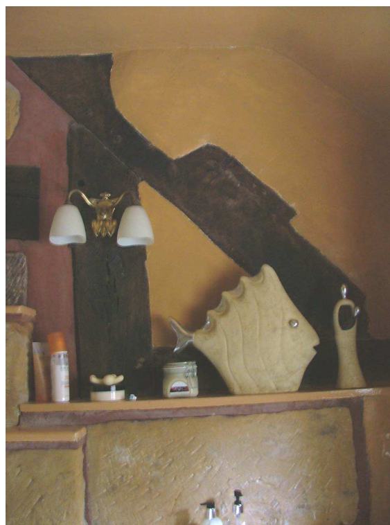
Plate 31 – Western side of former roof truss showing notch for former purlin in outer edge of rafter, bathroom
