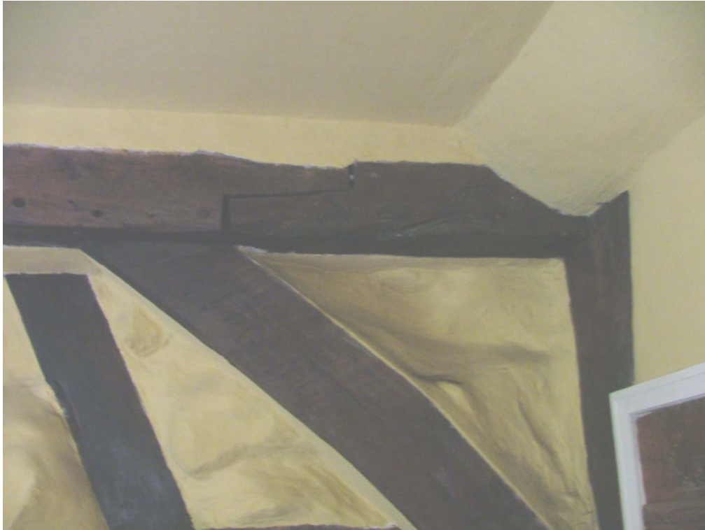
Plate 34 – Detail of scarf joint, east end of cross-wing timber frame, first floor bedroom
