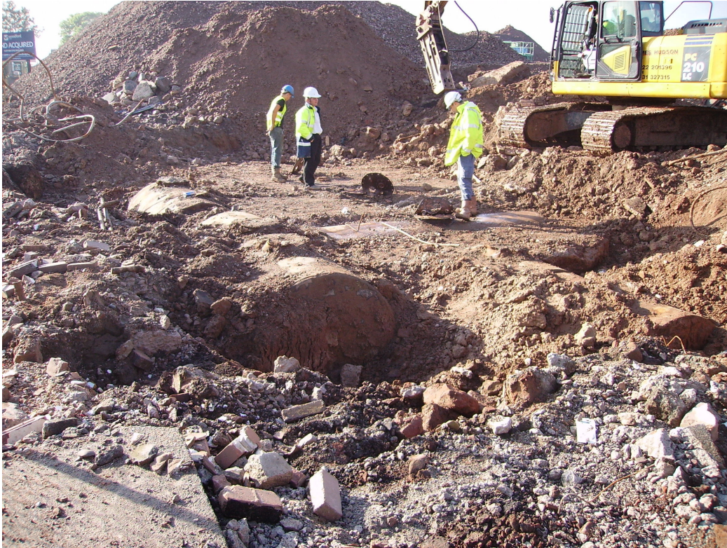
Plate 1: Underground Fuel Tanks
