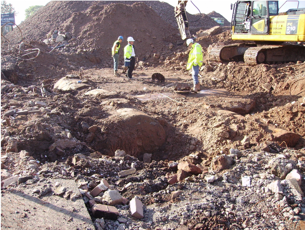
Plate1. Underground Fuel Tanks
