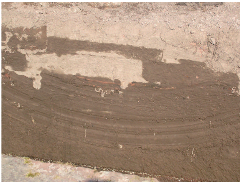
Plate 15: Scarring on the west side of wall 298
