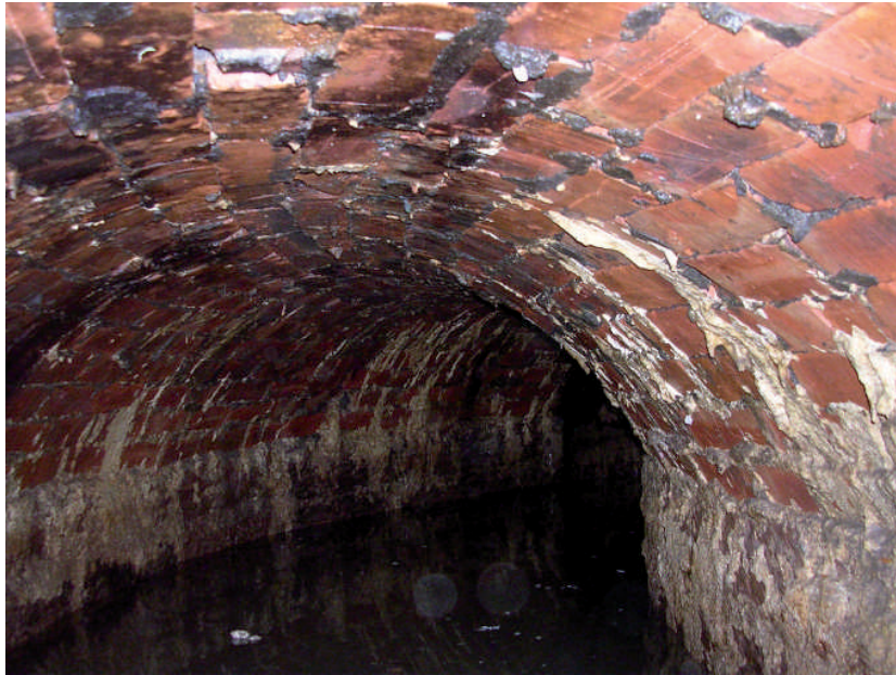
Plate 16: The brick arched tunnel leading from Wheel Pit B to condenser chamber
