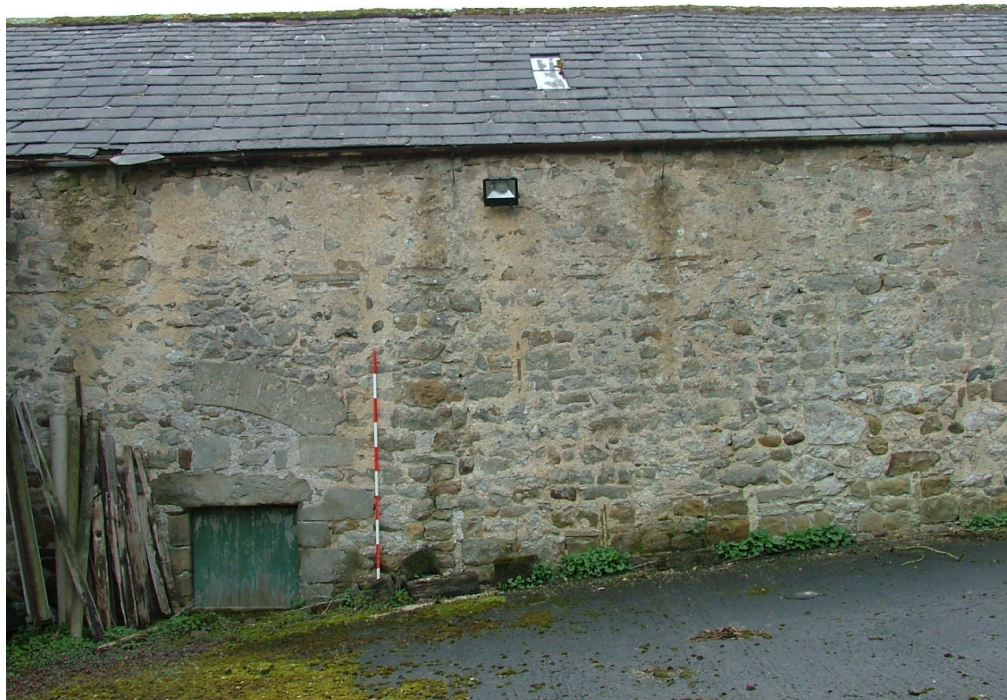
Plate 9 – Part of the north-west elevation showing the remains of a segmental arch and the blocked ventilation slits
