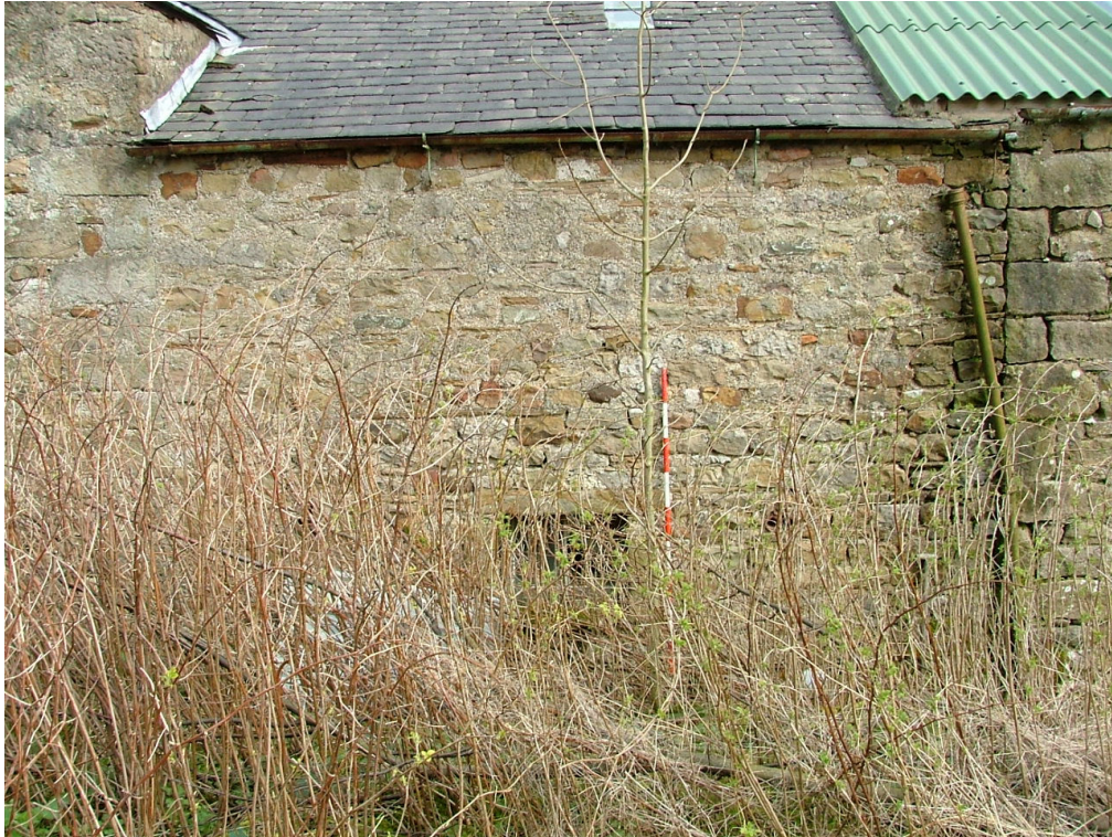
Plate 20 – South-west elevation of former granary/cowhouse showing two vertical construction breaks; one between Range A (left of photograph) and the other between the remainder of Range B (right of photograph)
