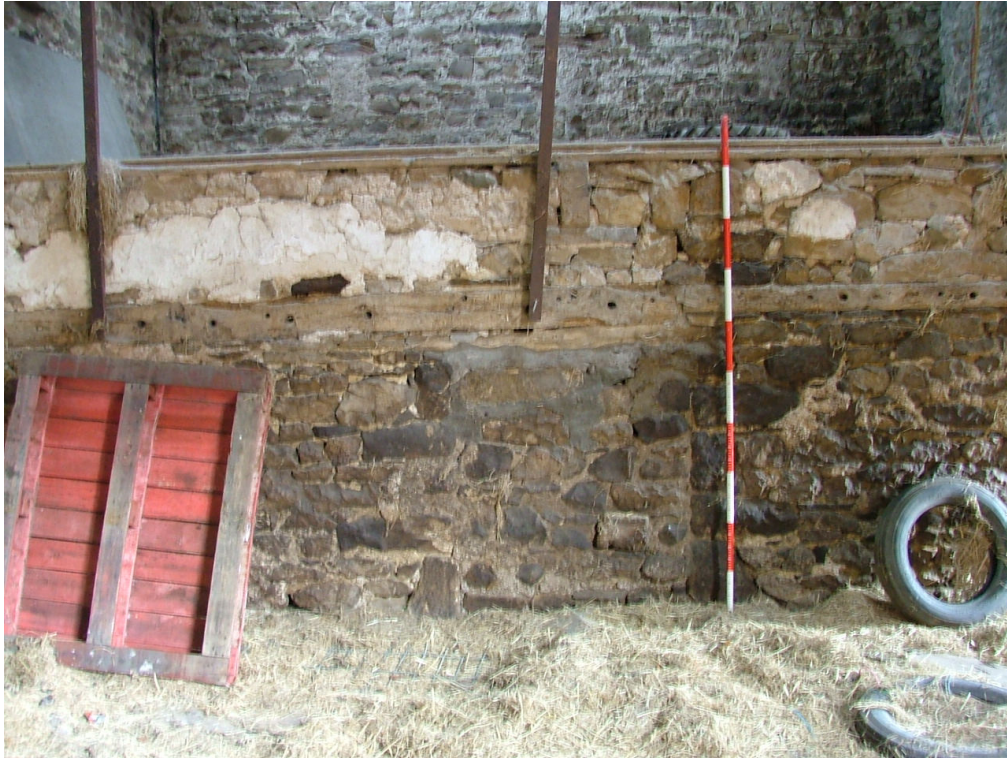
Plate 12 – Blocked hole in cross wall, north end of Range A (Scale = two metres)
