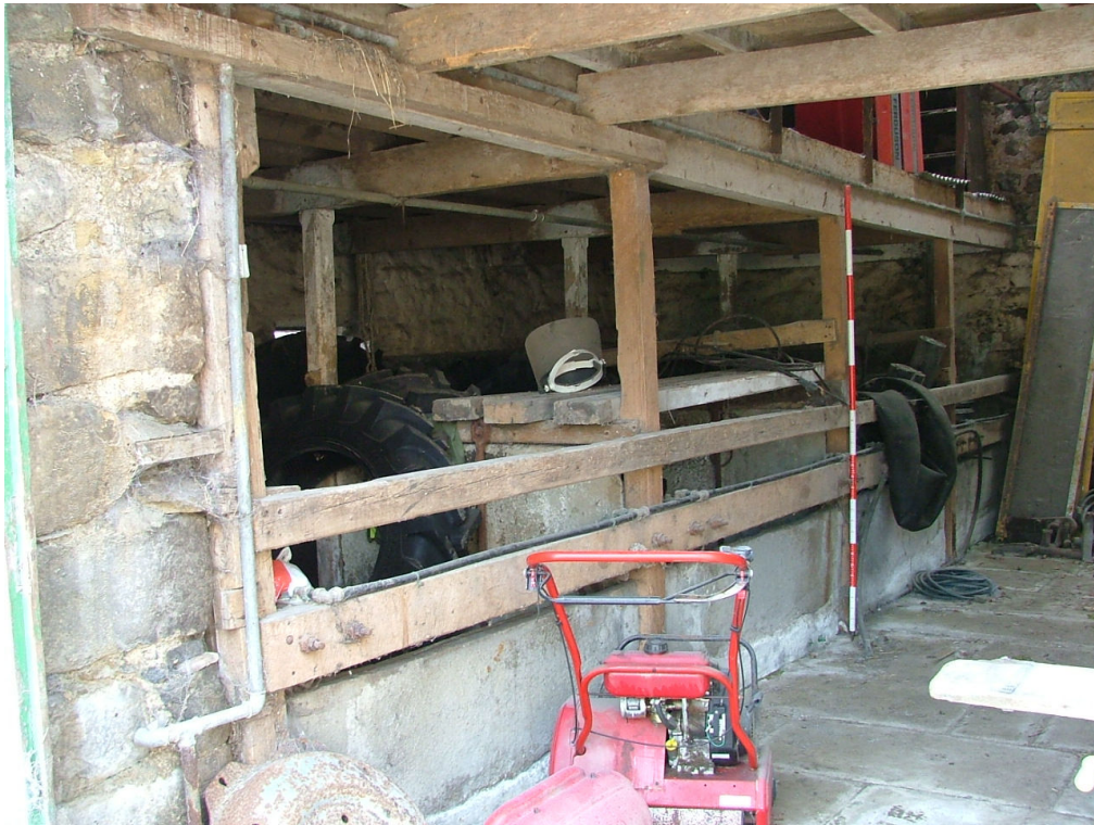
Plate 28 – Interior of large building, Range B showing stone and timber stall divisions and stone flagged floor of central section
