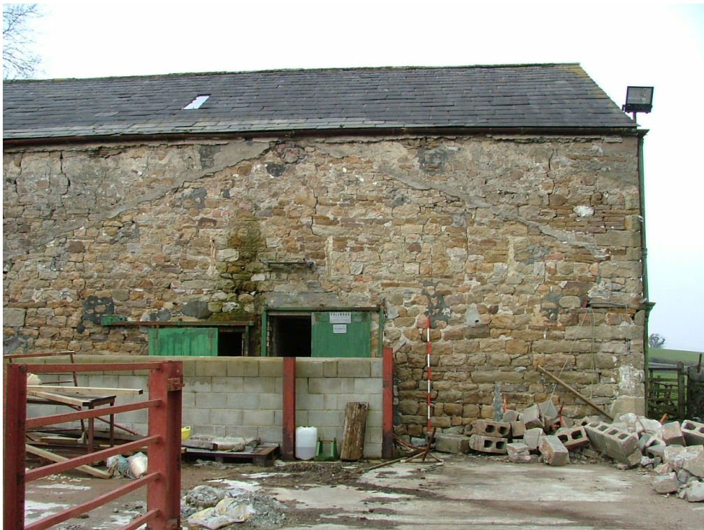
Plate 5 – South-east elevation of Range A showing blocked-up ventilation slits (Scale = two metres)
