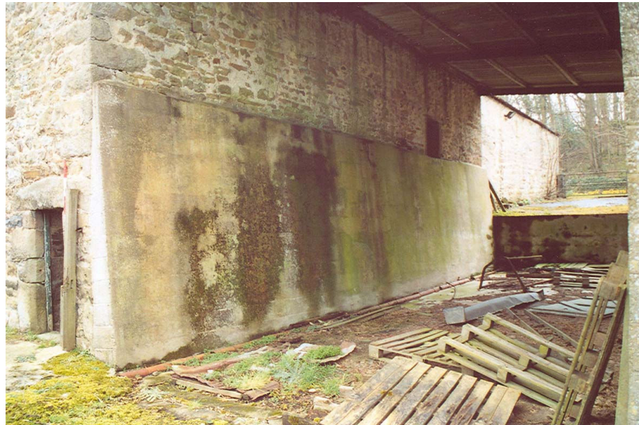
Plate 8 – Part of the north-west elevation obscured by the silage clamp, note the pitching hole to the right of photograph
