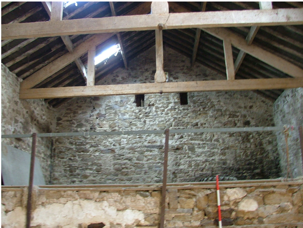
Plate 11 – Northern end of Range A showing the cross wall which creates a hayloft over the cow shed and root store
