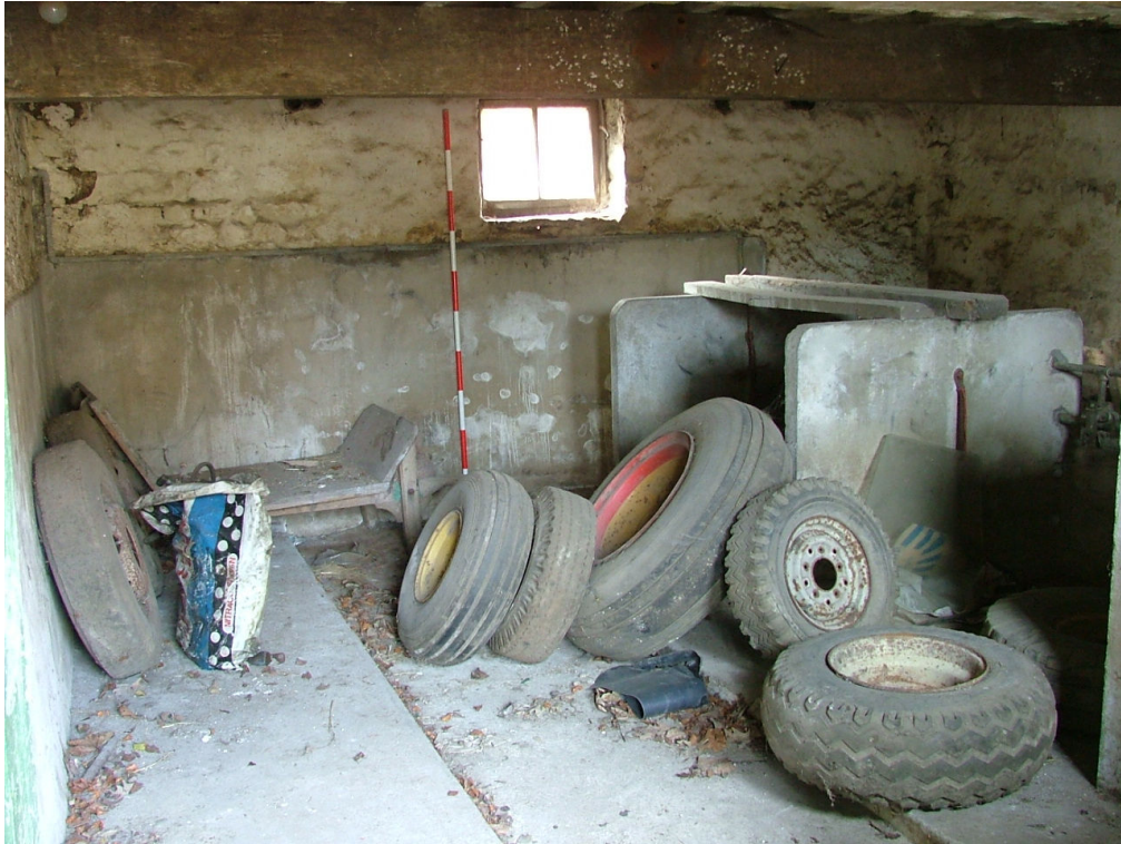
Plate 22 – Interior of cowhouse, Range B, showing concrete stall dividers, concrete floor and window in south-west elevation
