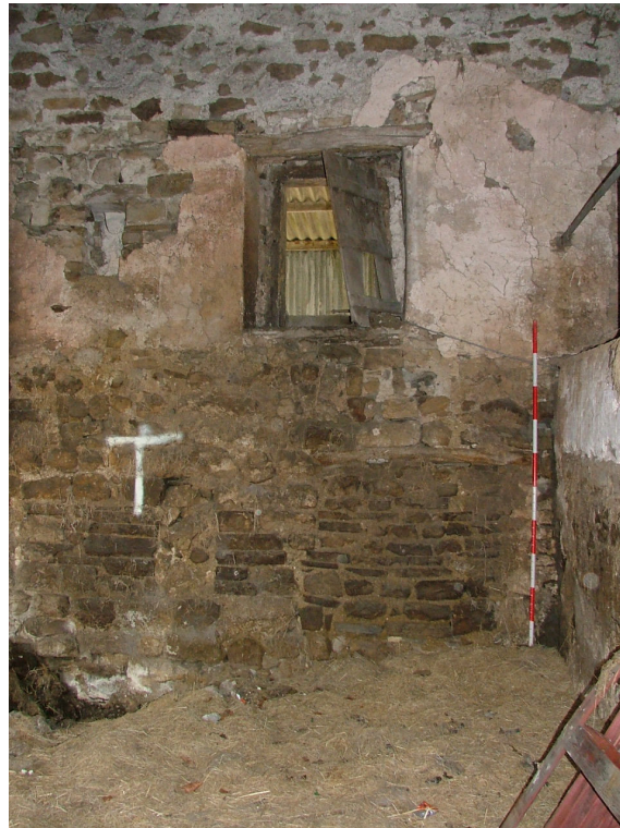
Plate 14 – Blocked doorway and pitching hole, north-west elevation of Range A
