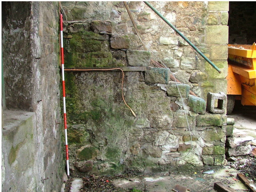
Plate 19 – Stone staircase to possible granary, Range B (built against the south-east elevation of Range A) (Scale = two metres)
