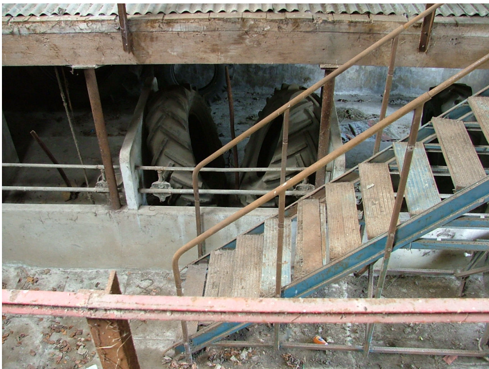
Plate 29 – Concrete stalls, right-hand side of main doorway, Range B, as seen from floor above
