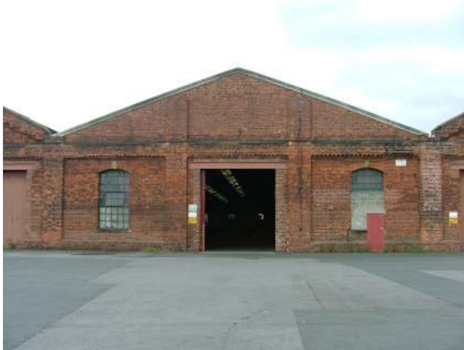
Plate 5 – Central section of south-east elevation showing lack of crow-step brickwork and circular window in gable. One window has had a door inserted and the large entrance is the original doorway for the engines
