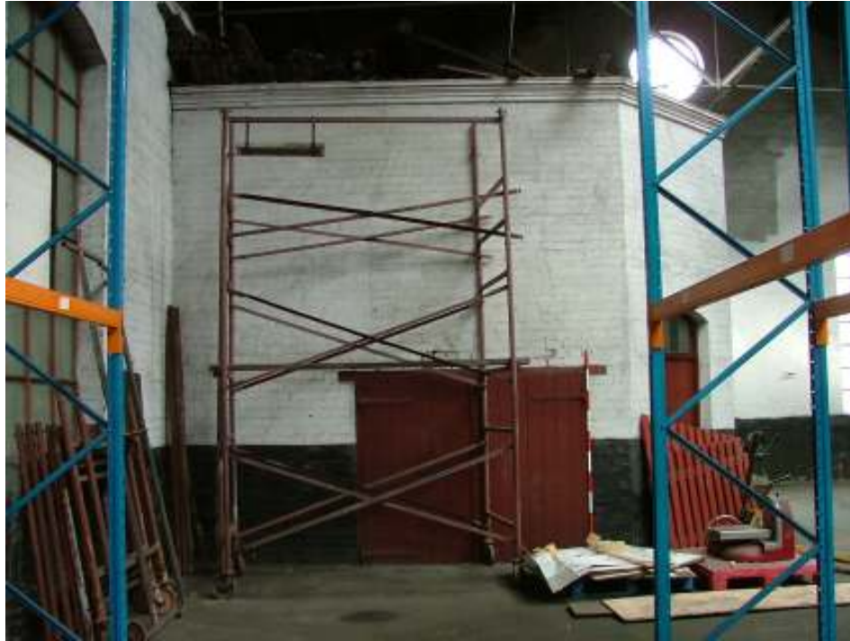
Plate 16 – Office in north-west corner of engine shed showing low doorway in south-east facing wall
