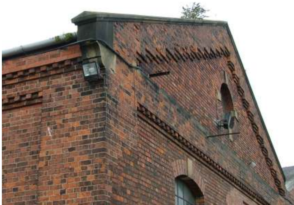
Plate 4 – Detail of the brickwork and sandstone coping stones and profiled kneeler (above the light), and dentilated brickwork below eaves and at the base of the panel below the gables, south-west elevation
