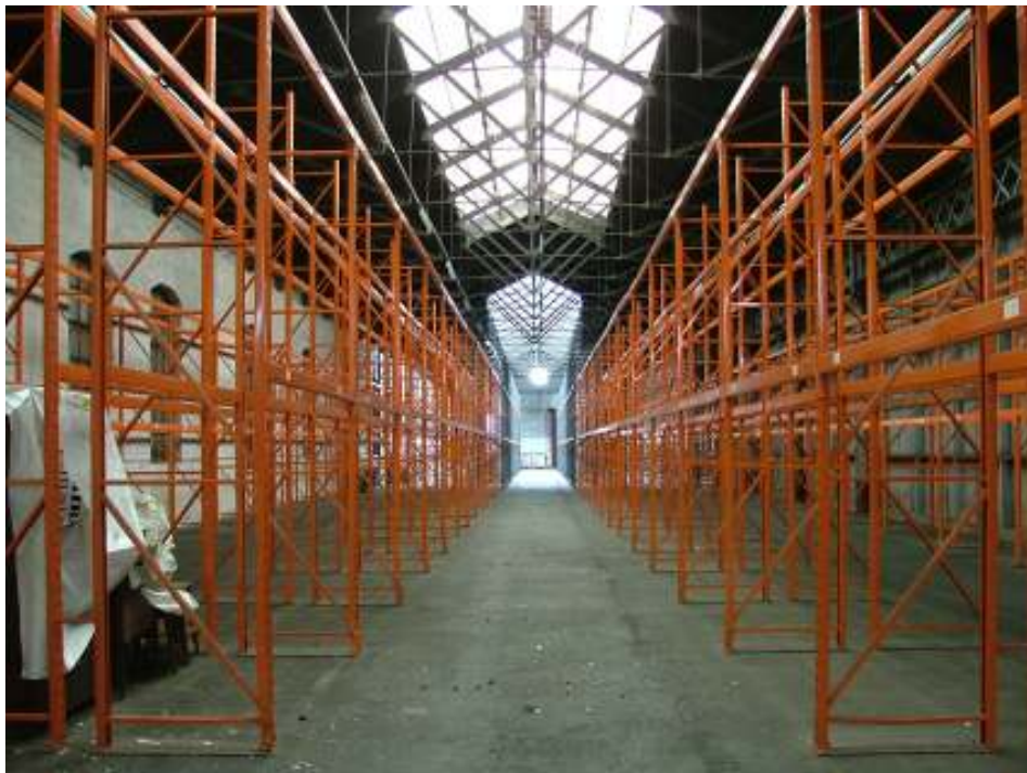
Plate 25 – View looking northwards of the western part of the shed showing roof structure including the raised sections, which provide extra light to the building
