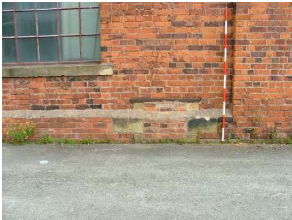
Plate 10 – South-west elevation, feature at base of wall (Scale is in 20cm graduations)
