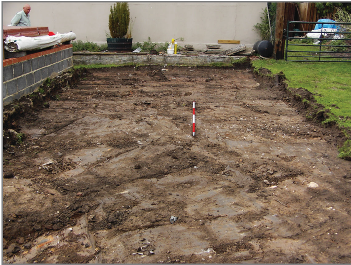
Plate 2. Northern section of site beyond pool area, showing limit of depth of excavation.
