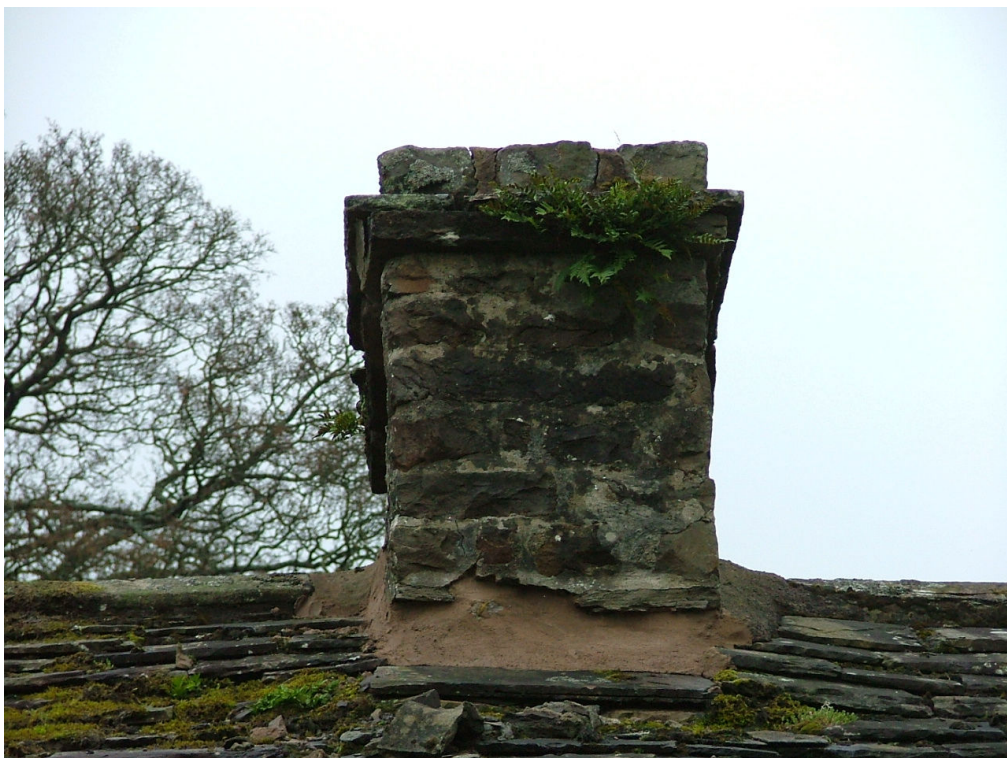
Plate 18 – Detail of chimney stack, mid-way along ridge showing modern mortar at base
