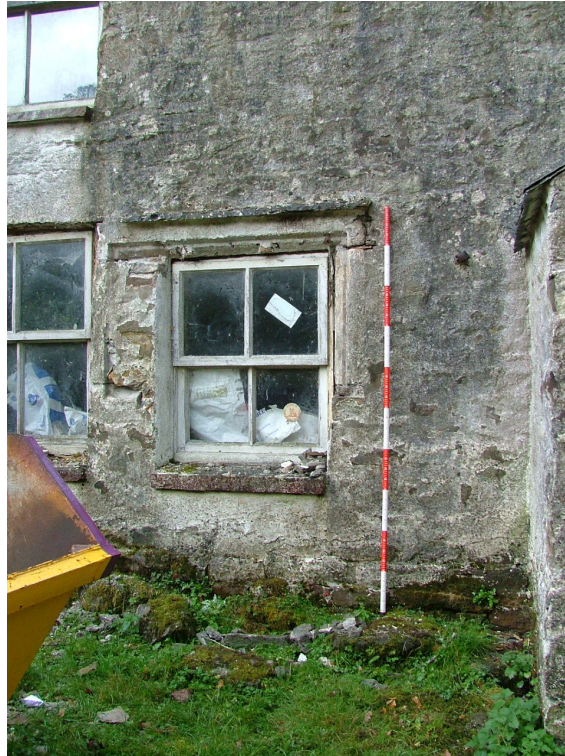
Plate 6 – Ground floor window to left of porch on south elevation showing earlier 3-light mullioned window and hoodmould (Scale = 2m)
