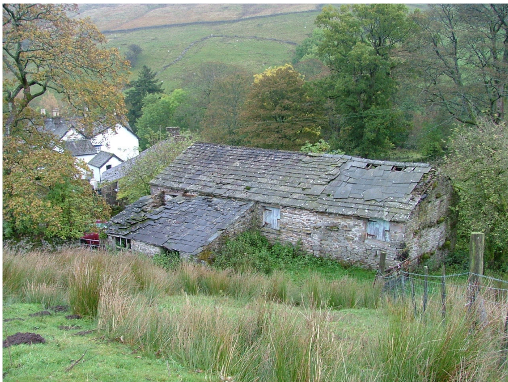
Plate 35 – Farm buildings to the south-west of the farmhouse as seen from the higher ground to the west
