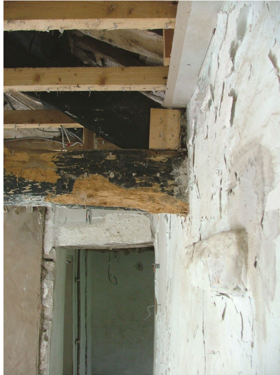
Plate 28 – First floor, view of through-stone and end of roof truss, north wall
