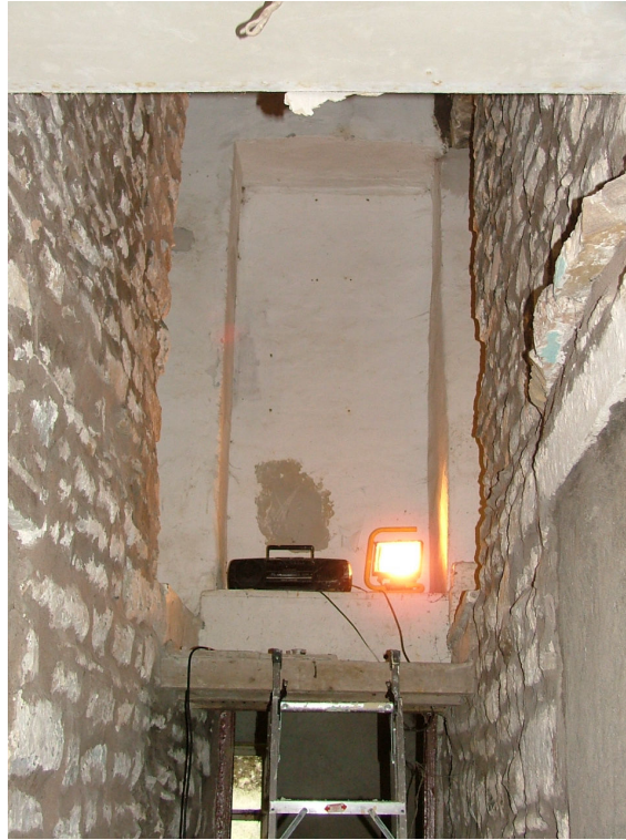
Plate 19 – Blocked-up first floor doorway as seen from bottom of stairwell looking north
