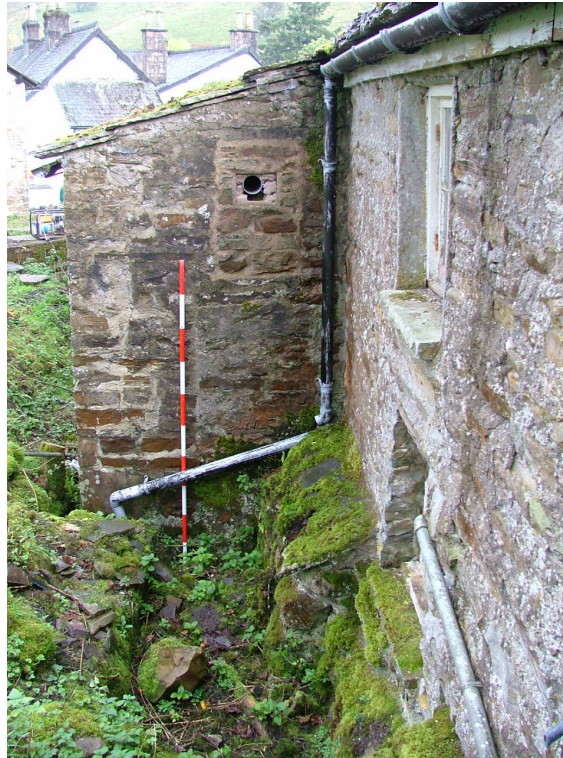
Plate 12 – Possible blocked window and modern blocked feature? West elevation of outshut to the rear of the house
