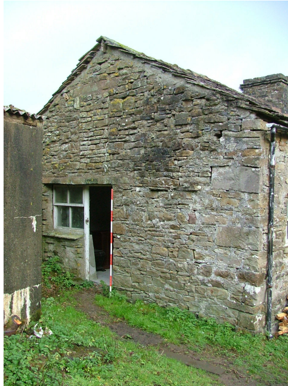
Plate 15 – West elevation showing doorway, window and first floor window now blocked (Scale = 2m)
