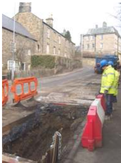
Plate 9: Excavation of trench, facing northwest, with the small test-pit in the background
