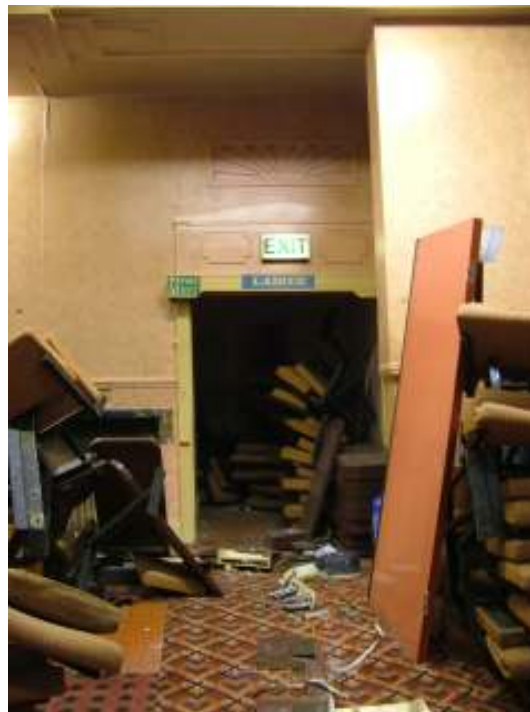
Plate 25 – Doorway at back of auditorium providing access to a fire escape, toilets and a door to the basement
