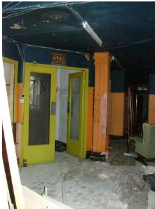
Plate 31 – View looking back towards the doors to the balcony foyer showing the stylised Ionic column
