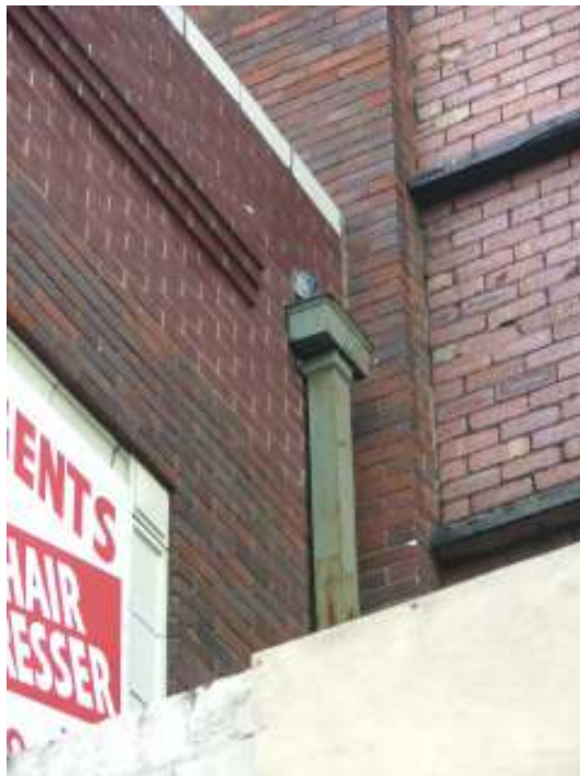
Plate 8 – Rainwater hopper and downpipe, east wall of first floor projection which houses the foyer for the balcony area of the cinema
