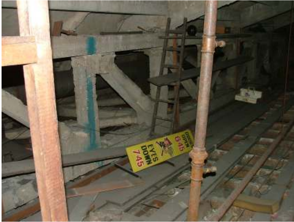
Plate 40 – View of the underneath of the balcony area showing the concrete construction. Note the sign for the bingo
