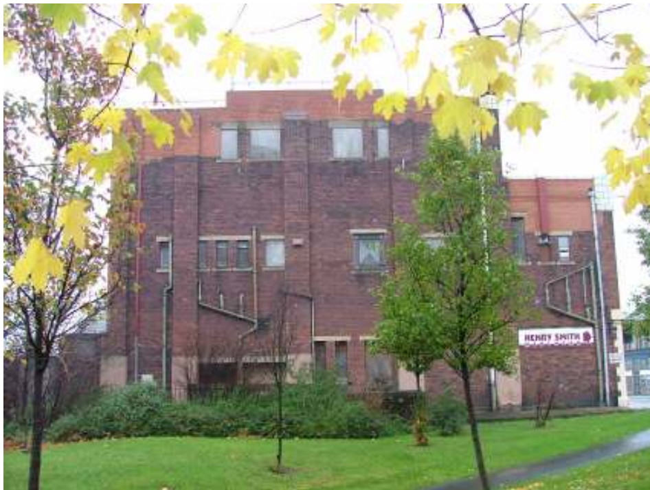
Plate 10 – West elevation of the Glenroyal Buildings showing the lack of architectural detail and areas of different coloured brick
