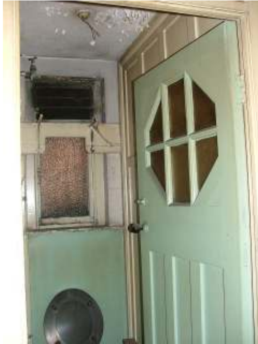
Plate 38 – View of the interior of one of the ladies toilets on the first floor
