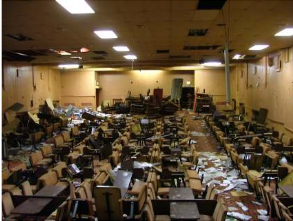
Plate 20 – View looking west of the main auditorium as seen from the stage
