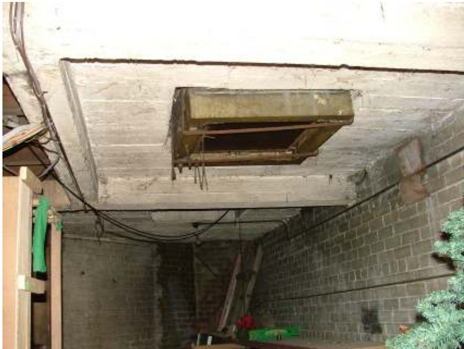
Plate 27 – View of the underside of the stage showing the concrete supported on brick walls and a metal duct?
