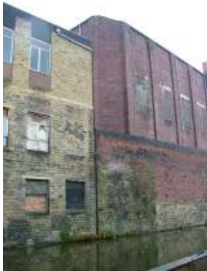
Plate 12 – View from the opposite side of the Leeds-Liverpool Canal, showing the north-east corner of the building, also note the brickwork making up the boundary wall constructed on earlier masonry walls
