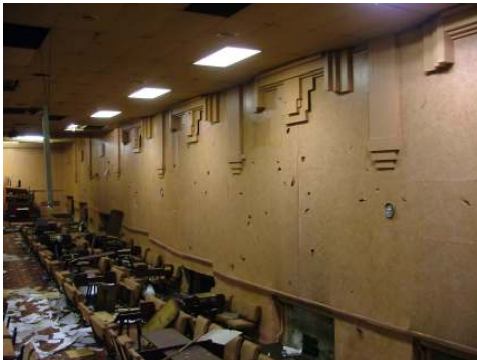
Plate 23 – North wall of the auditorium showing the base of the architectural detail, the rest of which is hidden by the suspended ceiling
