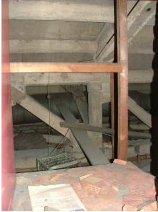
Plate 42 – View of the underneath of the balcony with large pipe visible in background
