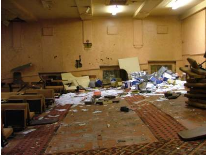
Plate 24 – View looking south of main auditorium showing the location of some of the radiators, and the scarring in the floor boards where the former seating were located
