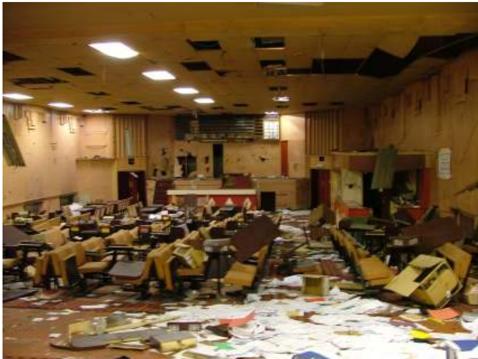
Plate 19 – View looking east towards the stage of the main auditorium showing the remaining seating for the bingo hall and the suspended ceiling
