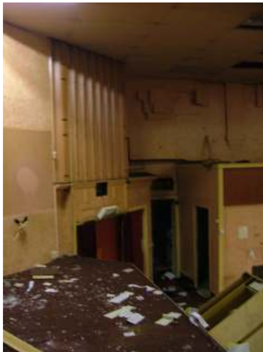
Plate 21 – View looking south from the stage showing the base of the proscenium consisting of vertical lines, over one of two fire exits which flank the stage
