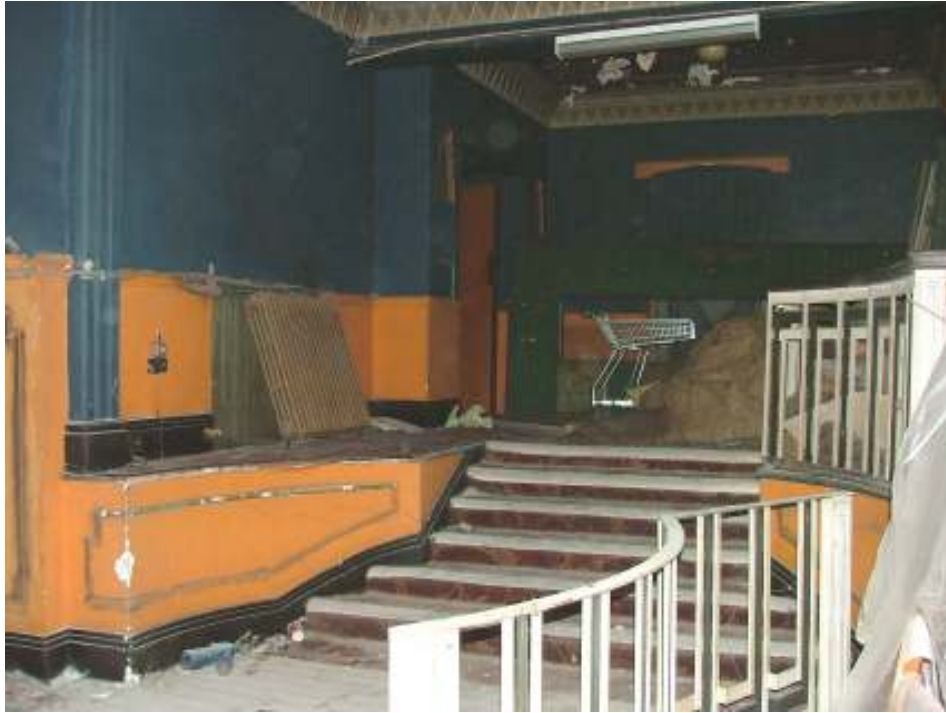
Plate 30 – Stairs to balcony from the first floor foyer, showing blue and gold décor, decorative ceiling and black and white iron balustrades
