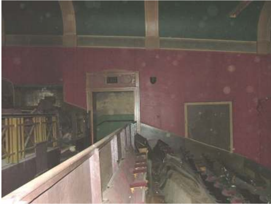
Plate 34 – View of the balcony area showing the original seating still in-situ , the doorway provides access to the emergency fire exit down the external staircase
