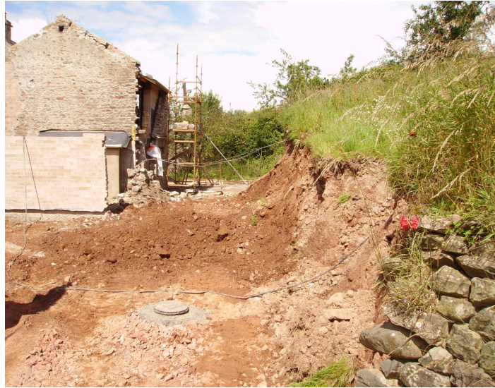
Plate 7: Excavation into the bank at the rear of Barn A. Note that the majority of the rear wall has been demolished.
