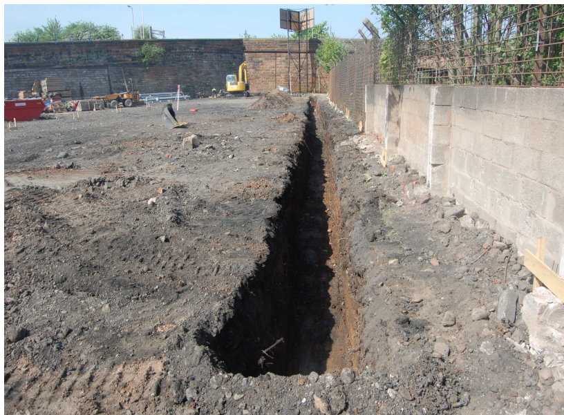
Plate 1: Excavation of the foundation trench northern extent of the site, facing west
