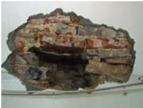
Plate 6: Hole inserted in west wall of small room north of the lobby
