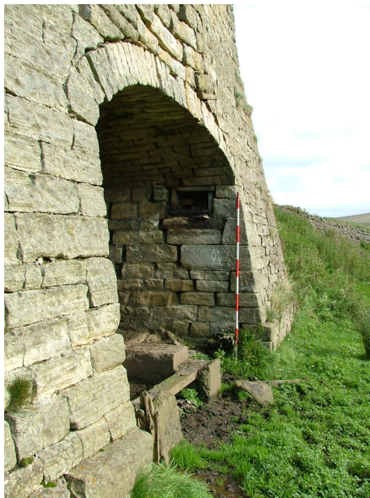
Plate 7 – Right-hand draw arch, showing concrete blocks and wood-lined hole for former pulley (Scale = 2m)
