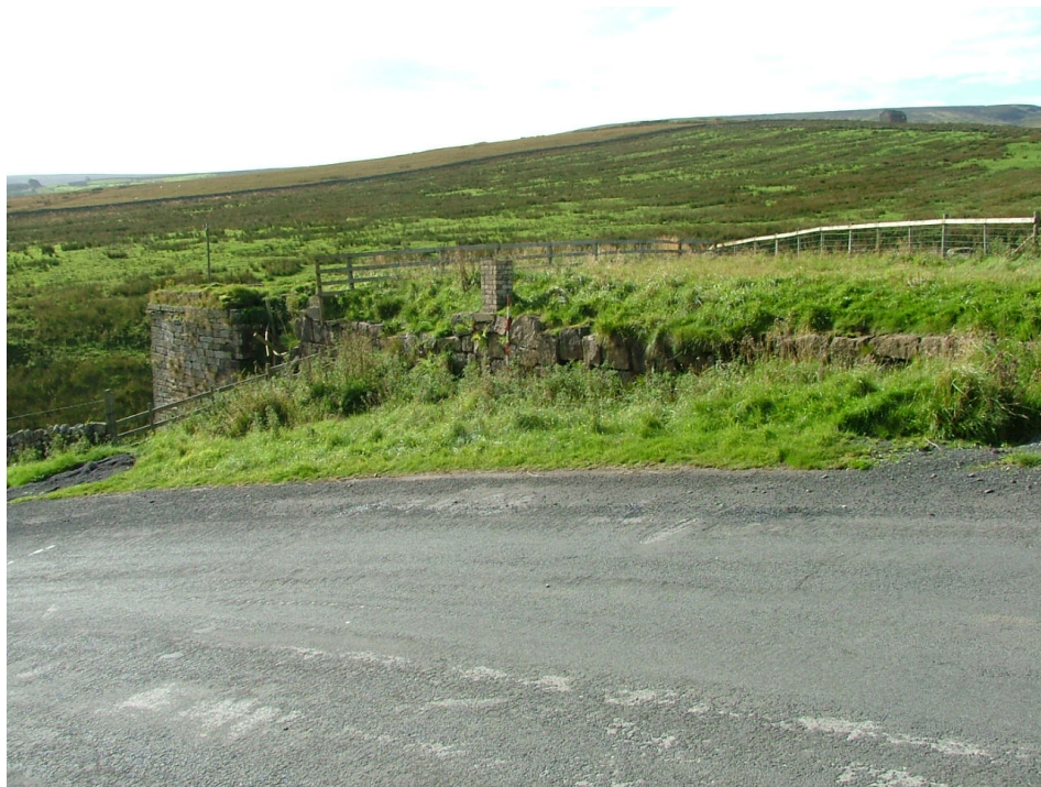
Plate 12 – View looking south from the road showing the level ramp leading to the top of the limekiln and the retaining wall
