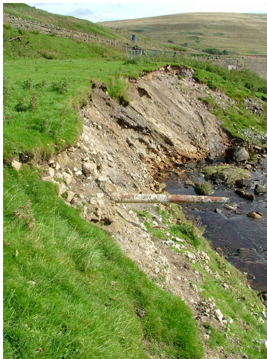
Plate 19 – View looking north-east showing the metal pipe protruding from the north bank of Middlehope Burn
