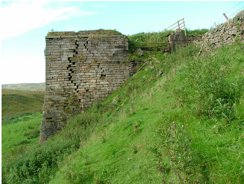
Plate 10 – North-east elevation showing structural defects (Scale = 2m)
