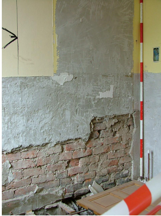
Plate 50 – Brick wall which separated the communal bathroom and the corridor, first floor (Scale is in 20cm graduations)
