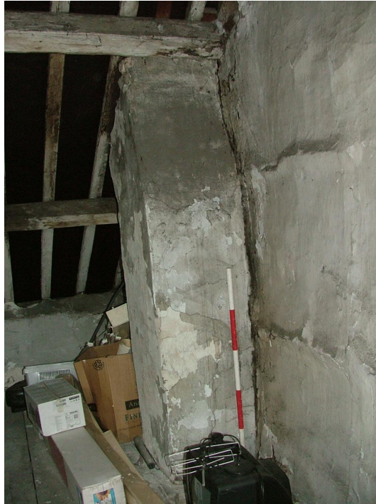
Plate 38 – South-western brick chimney stack in attic (Scale = 1m), note the lack of bonding to the wattle and daub wall
