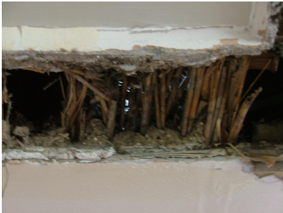
Plate 66 – Layer of dried reed stalks within ceiling between Bedroom 1 and the hall on the second floor
