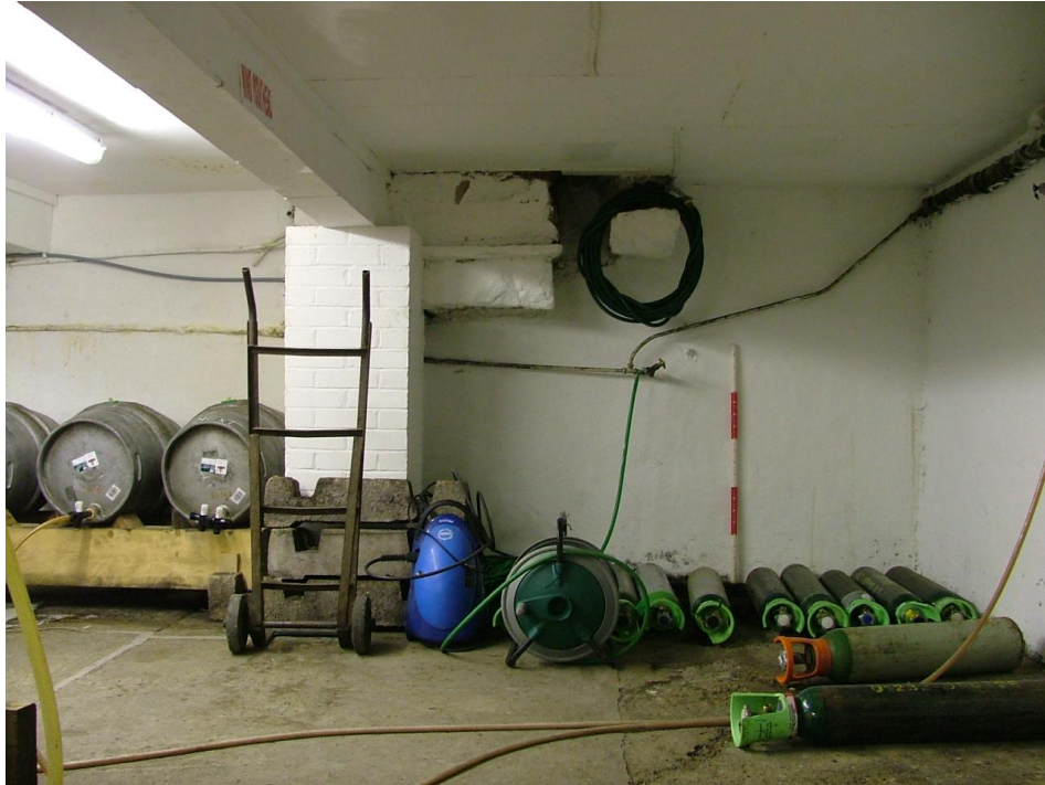
Plate 24 – Brick support pier for girder and remains of projecting masonry, south-east wall of cellar (Scale = 1m)
