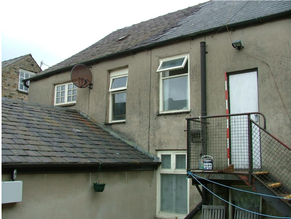
Plate 16 – South-west elevation of Wagon and Horses as seen from the fire escape stairs (Scale = 2m)
