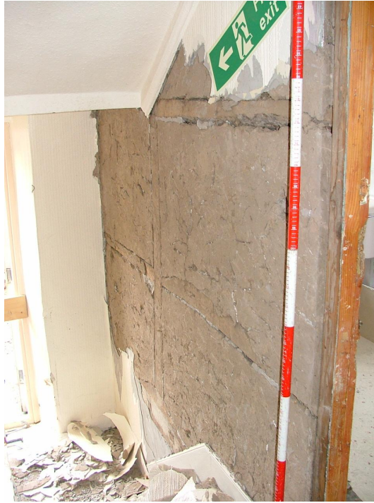
Plate 54 – Timber-framed wall between bathroom and stairwell, second floor (Scale is in 20cm graduations)
