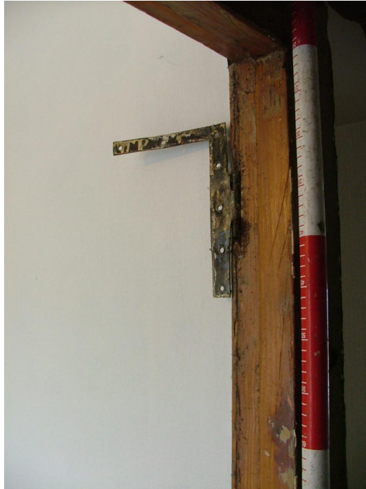
Plate 56 – L-shaped hinge in-situ on bathroom doorframe, second floor (Scale is in 1cm graduations)
