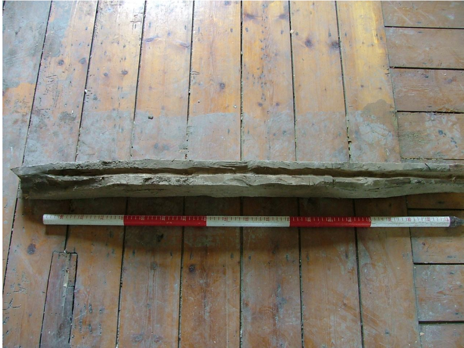
Plate 60 – Top side (showing shallow groove) of horizontal timber removed from timber-framed wall, second floor (Scale = 1m)
