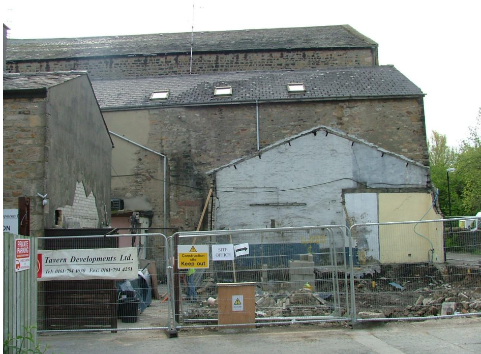
Plate 46 – View looking south-east of the rear of the Wagon and Horses after the demolition of the modern garage/workshop showing the scarring of the gable against the adjoining former warehouse
