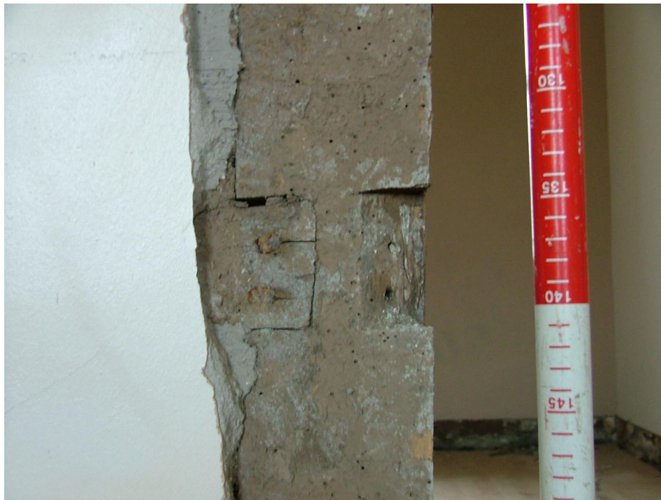
Plate 51 – Notch in left-hand timber of door surround, Bedroom 1, second floor (Scale is in 1cm graduations)
