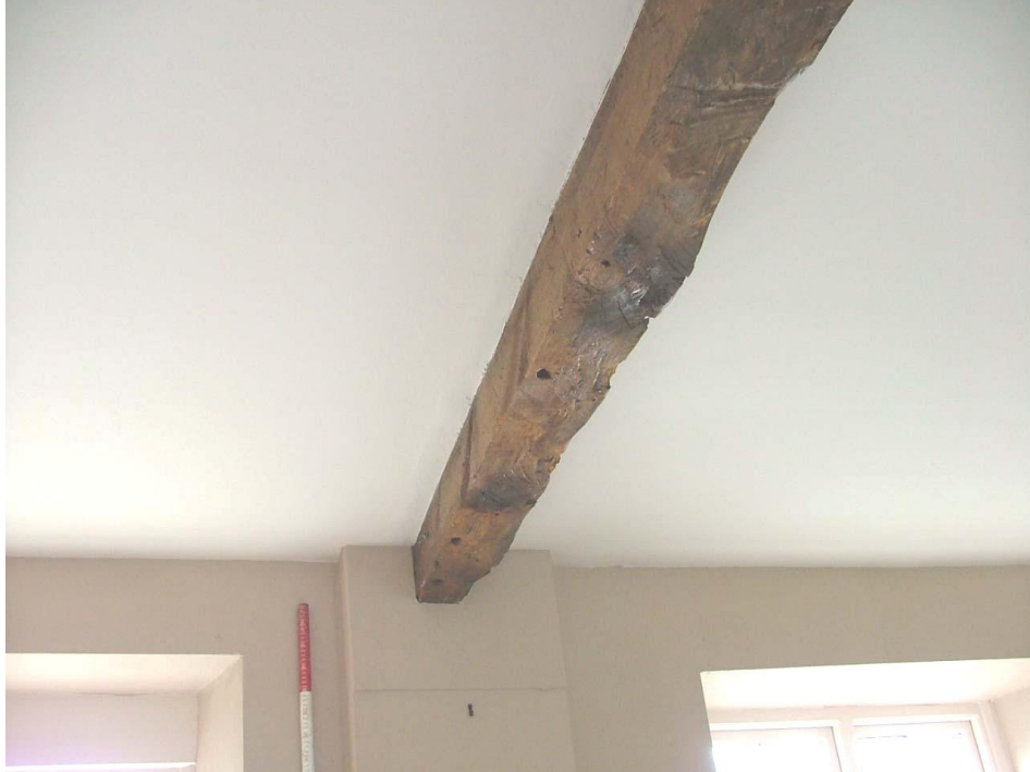
Plate 30 – South-west end of beam in living room (second floor) showing several circular holes possibly relating to an internal partition
