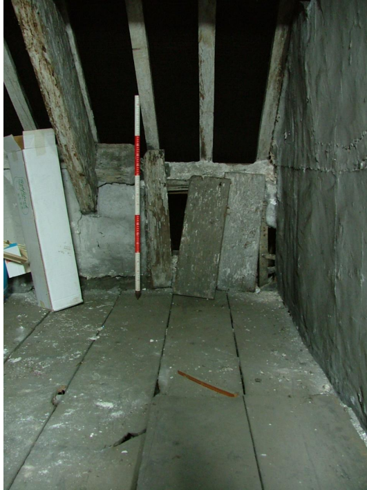
Plate 44 – The base of the rafters has a short wall which presumably preventing the wind blowing into the attic (Scale = 1m)
