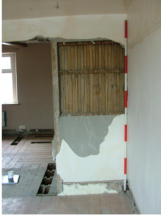
Plate 52 – Lathe and plaster section of wall between Bedroom 1 and the hall, second floor, this appears to have been inserted in the original location of the door into the room (Scale = 2m)
