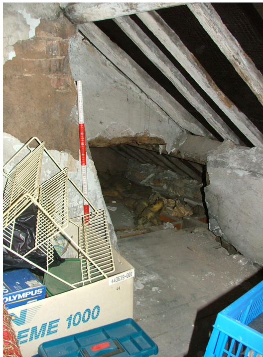
Plate 41 – Small hole in northern cross-wall in attic, possible modern insertion when the two properties became one (Scale = 1m)
