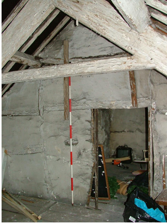
Plate 36 – View looking north of the southernmost cross-wall in the attic, showing the timber-framing with wattle and daub infill and door frame (Scale = 2m)
