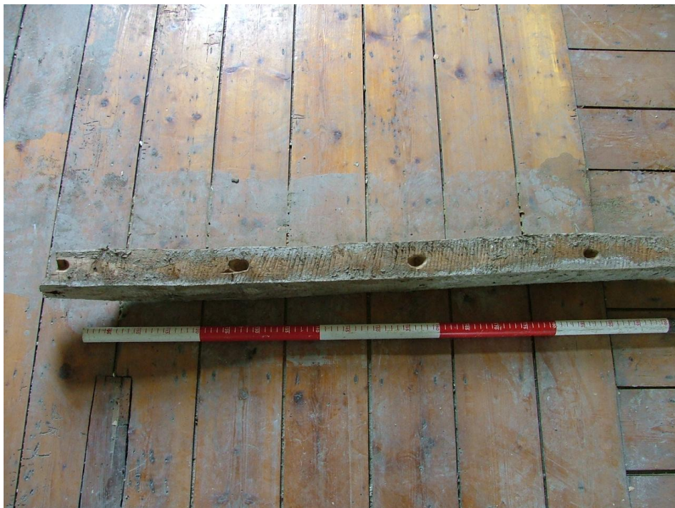
Plate 59 – Underside of one of the horizontal timbers removed from the timber-framed wall, second floor (Scale = 1m)
