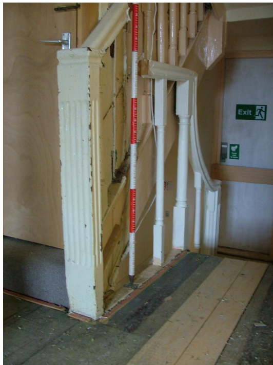
Plate 27 – Detail of newel post, balusters and ramped handrail of staircase as seen on the second floor (Scale is in 20cm graduations)
