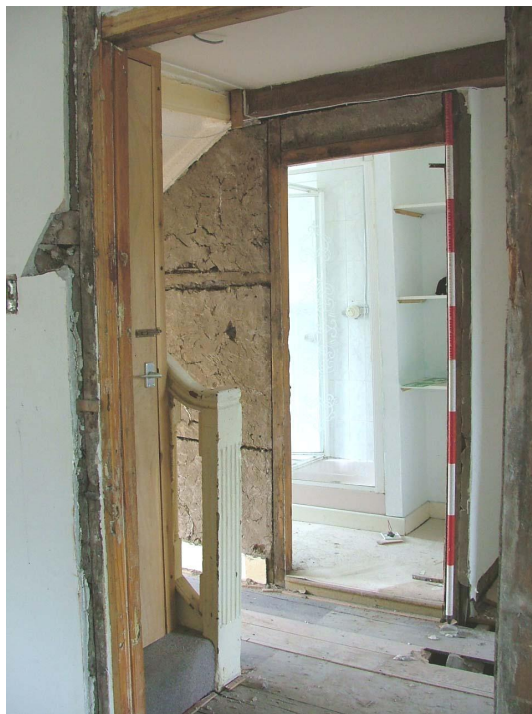
Plate 53 – Original timber-framed wall and door frame, bathroom on second floor (Scale = 2m)
