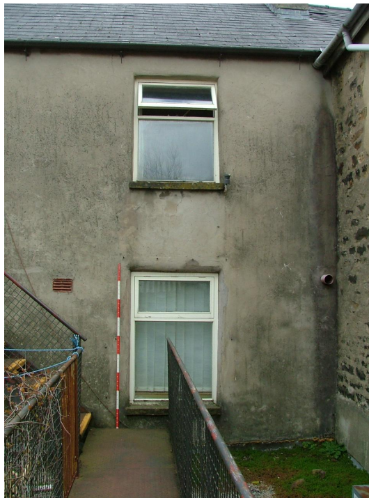
Plate 17 – Part of the south-west elevation as seen from the fire escape on the top of the single-storey extension which houses the toilets (Scale = 2m)
