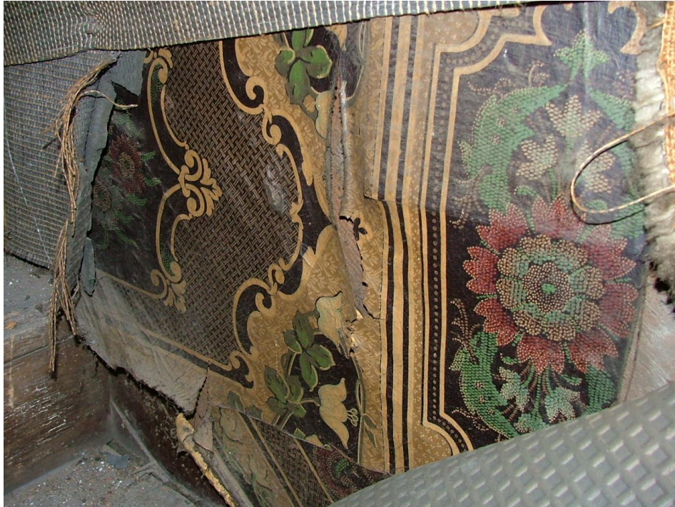
Plate 34 – Detail of the wallpaper largely hidden behind carpet underlay, right-hand side of staircase leading into the attic
