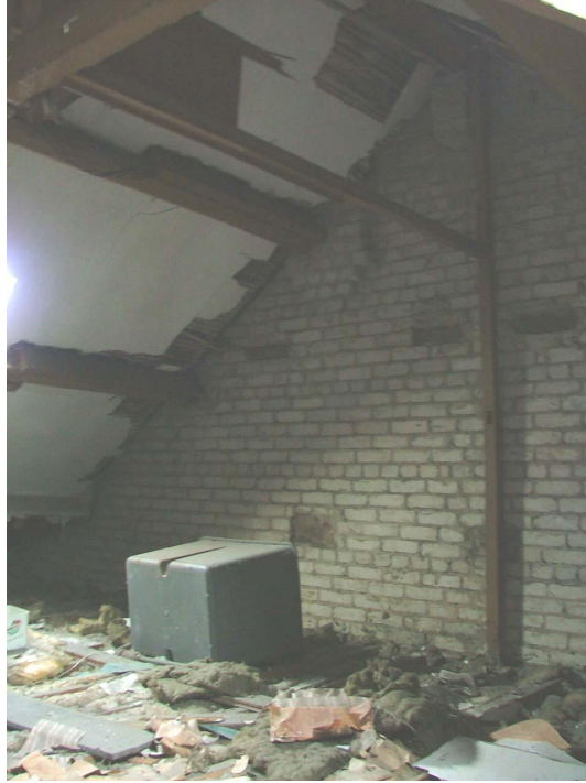
Plate 42 – North-west gable end as seen from the attic space showing brickwork of modern rebuild (it was not possible to include a scale in this photograph due to the lack of floorboards)
