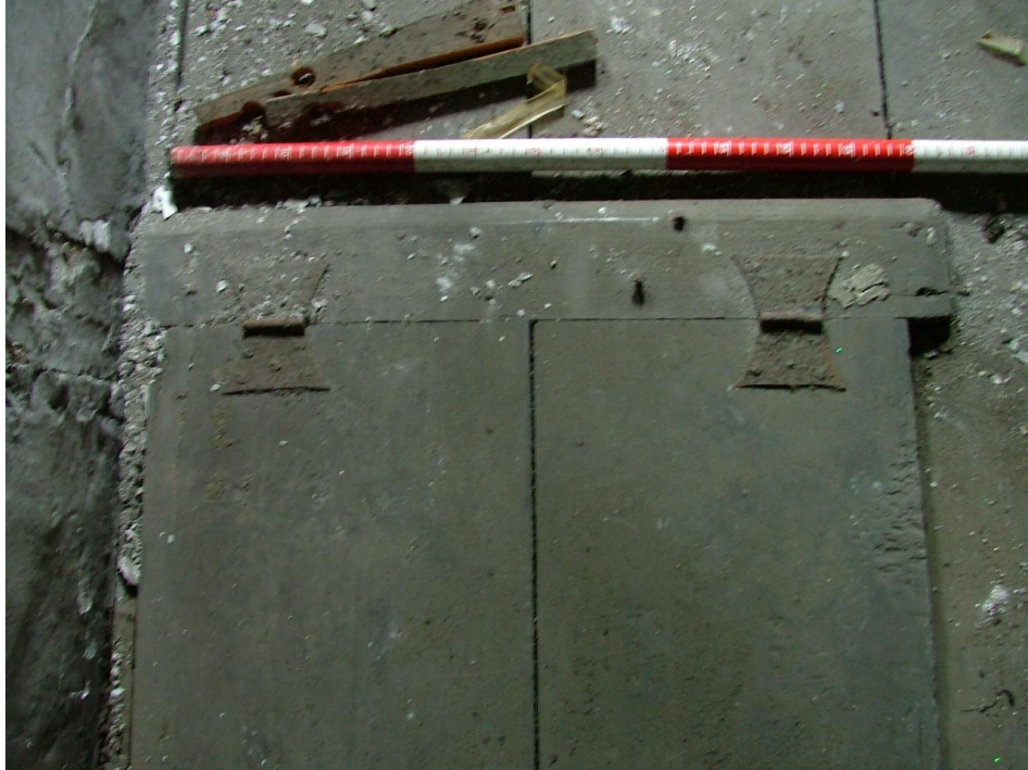
Plate 40 – Detail of the butterfly hinges, wooden hatch in attic floor (Scale is in 20cm graduations)
