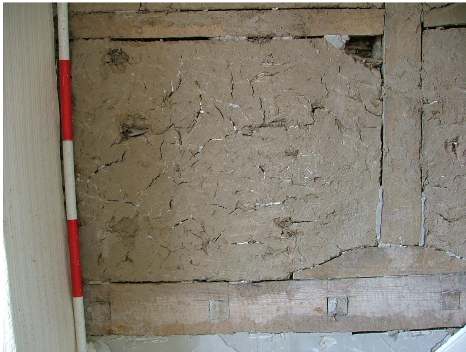
Plate 55- Base of timber-framed wall showing detail of construction (Scale is in 20cm graduations)
