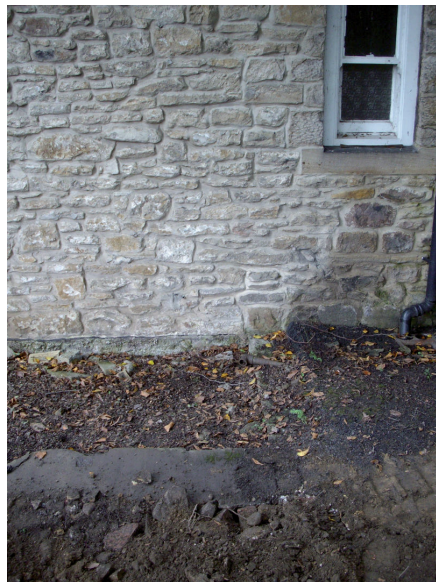
Plate 4: east-facing wall showing modern extension foundations butting against the base of the standing wall.
