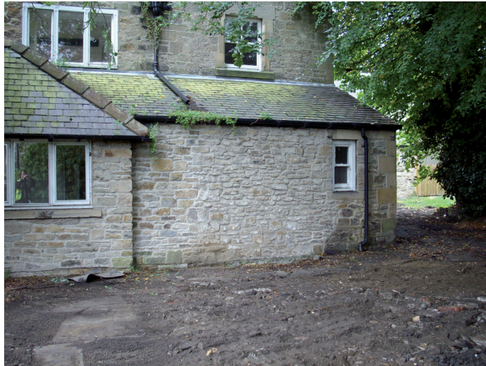
Plate 3: east-facing wall of East House, showing repairs to sandstone wall after demolition of modern outbuildings.
